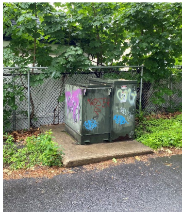
Utility Company Pad-mount Transformer
