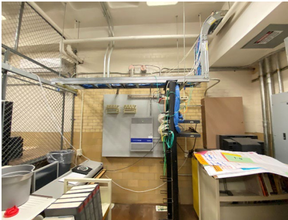
Telecommunications & Wire Cable Management
