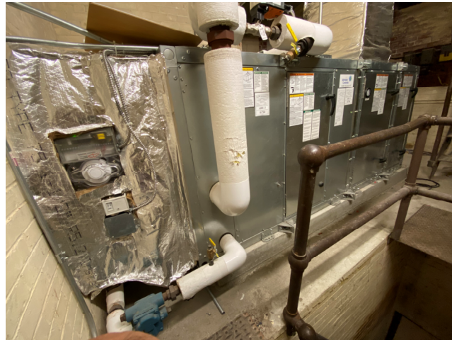
Photos 13 : Existing AHU serving the Auditorium.
