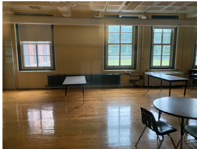
Photos 10: Typical classroom radiator and unit ventilator.
