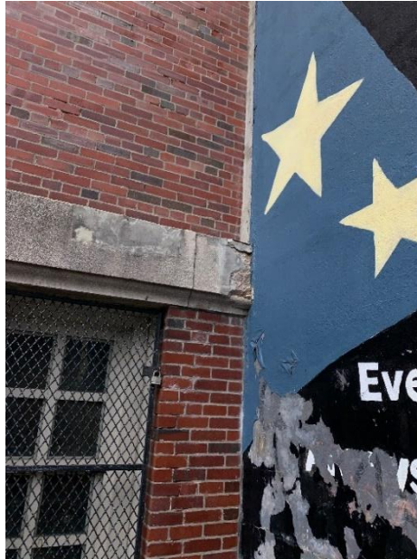
Spalled cast stone cornices and headers will require structural repairs or replacement.
