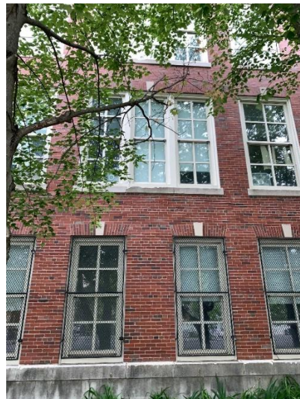
View of exterior portion of building showing large windows at level 2 where brick above is supported by continuous steel relieving angle. Structural repairs will be required.
