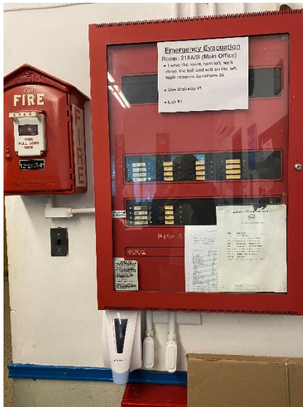
Fire Alarm Control Panel and Master Box
