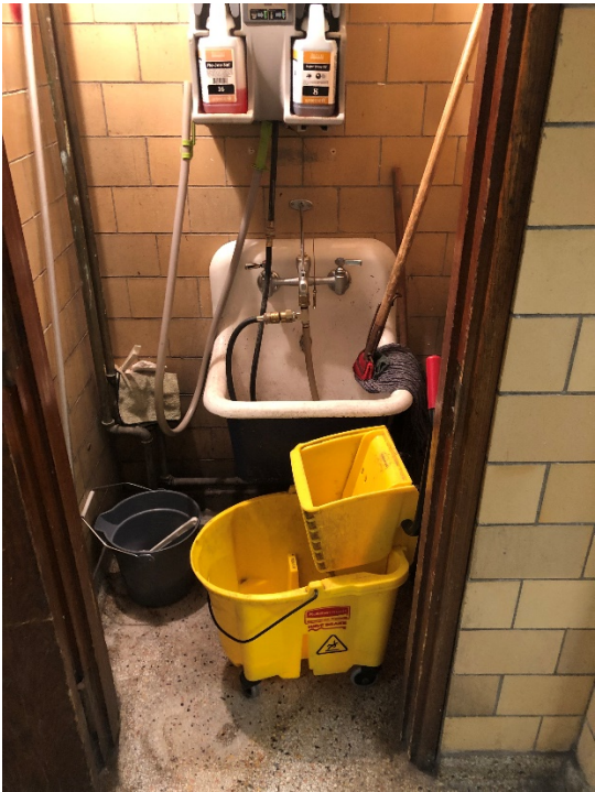
Photo 12: Cast Iron Mop Sink with Detergent Dispenser
