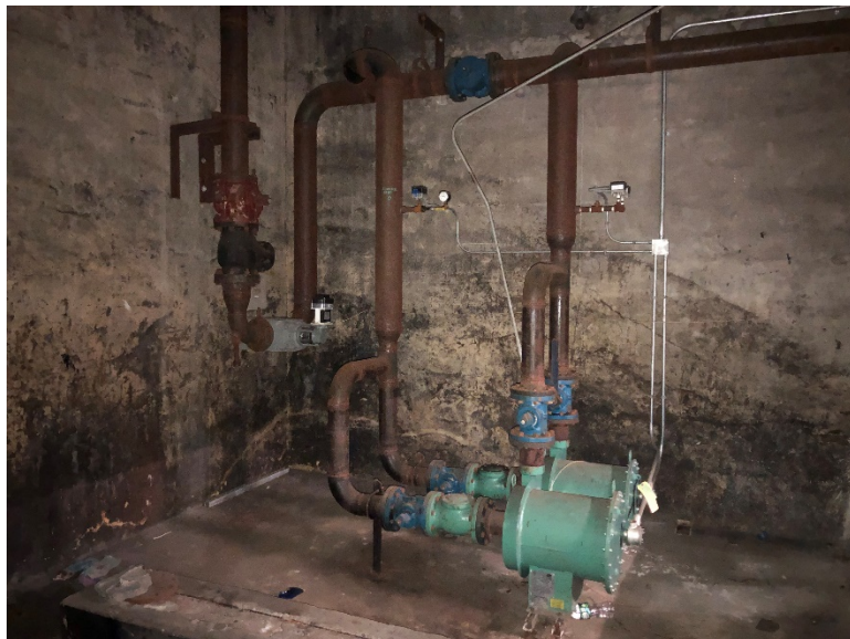
Photo 5: Gas Pressure Booster System
