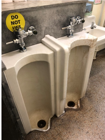
Photo 10: Floor Mounted Urinals
