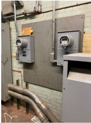
Main Disconnect Switch & Meters
