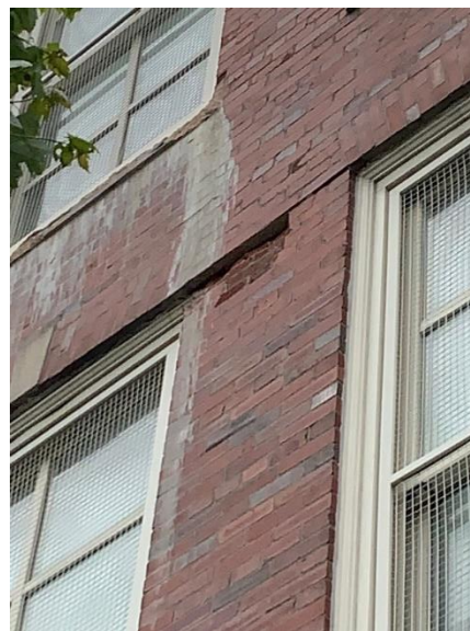
Major spalls and corroded relieving angle will require repairs / replacement.
