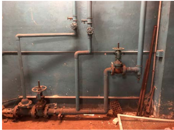
Photos 1 & 2: Domestic Water Service
