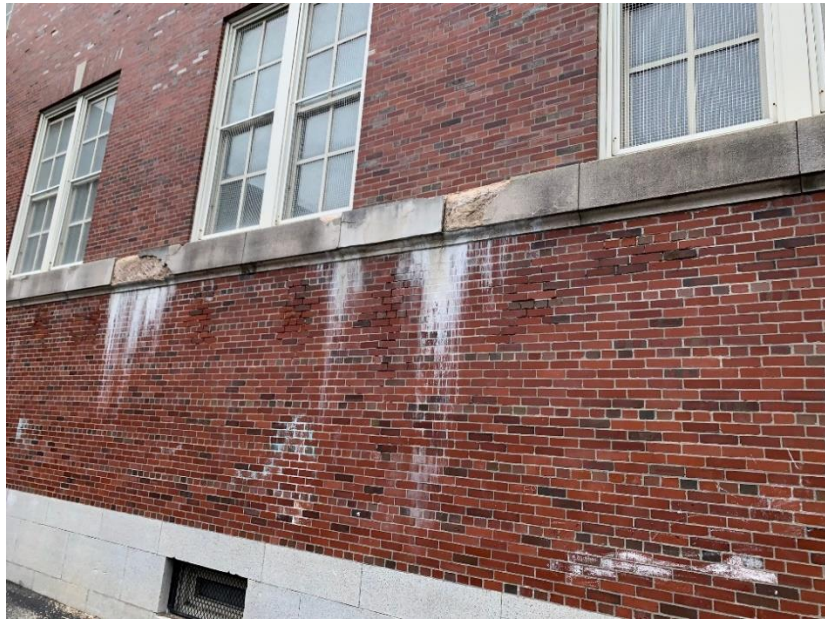
Spalled cast stone sills and deteriorated brick wall along exterior of building will require repairs / replacement.
