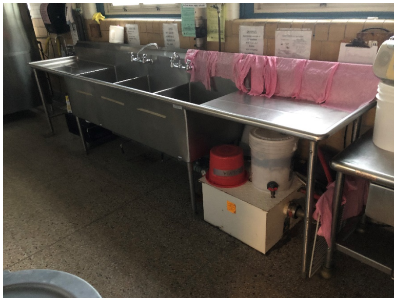
Photo 16: Scullery Sink & Grease Interceptor
