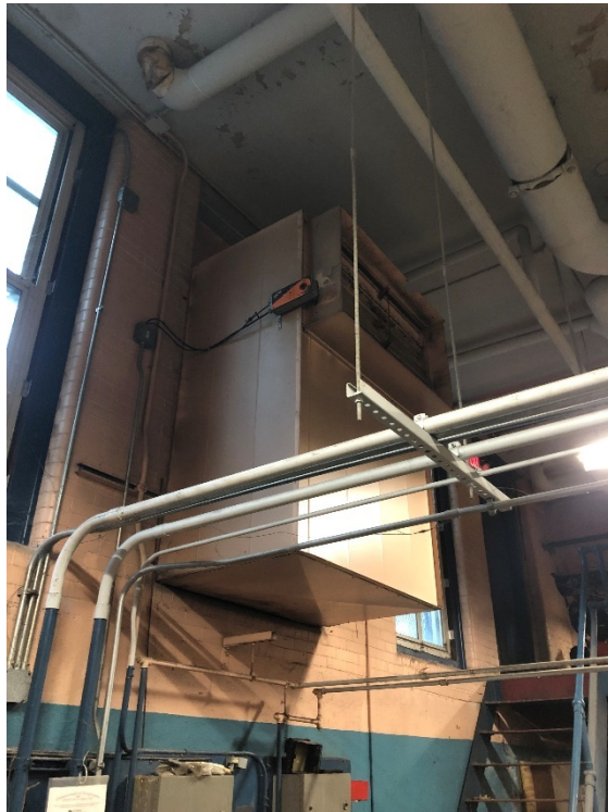
Photo 6: Combustion Air Duct
