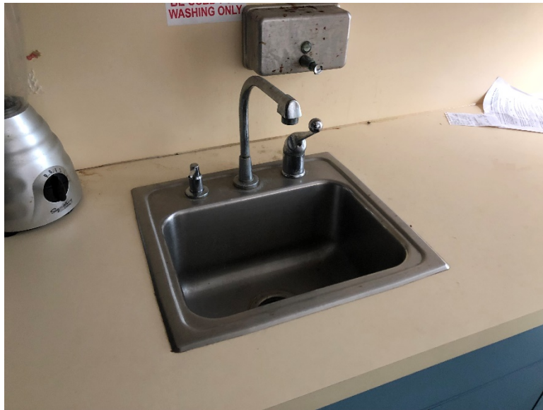
Photo 13: Typical General Use Sink
