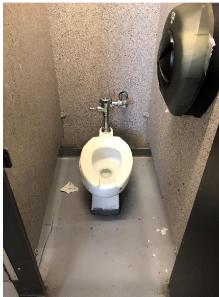
Photo 7: Typical Water Closet
