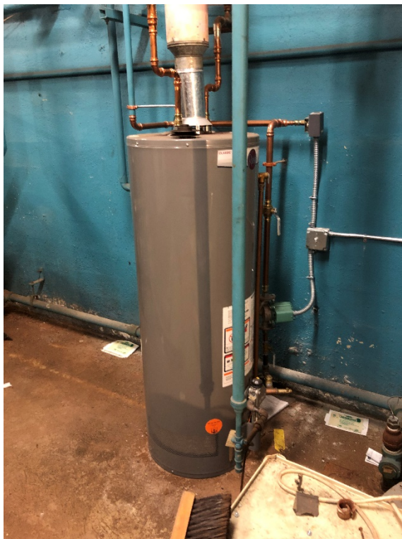
Photo 3: Gas Fired Water Heater
