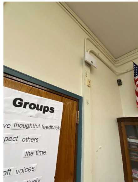
Wireless Access Point Devices
