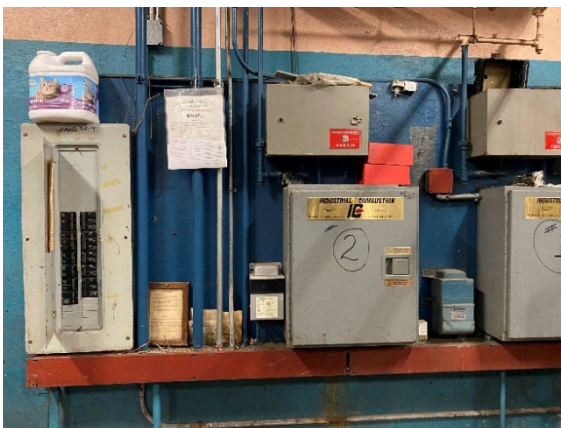
Feeder Circuit Breaker Panels
