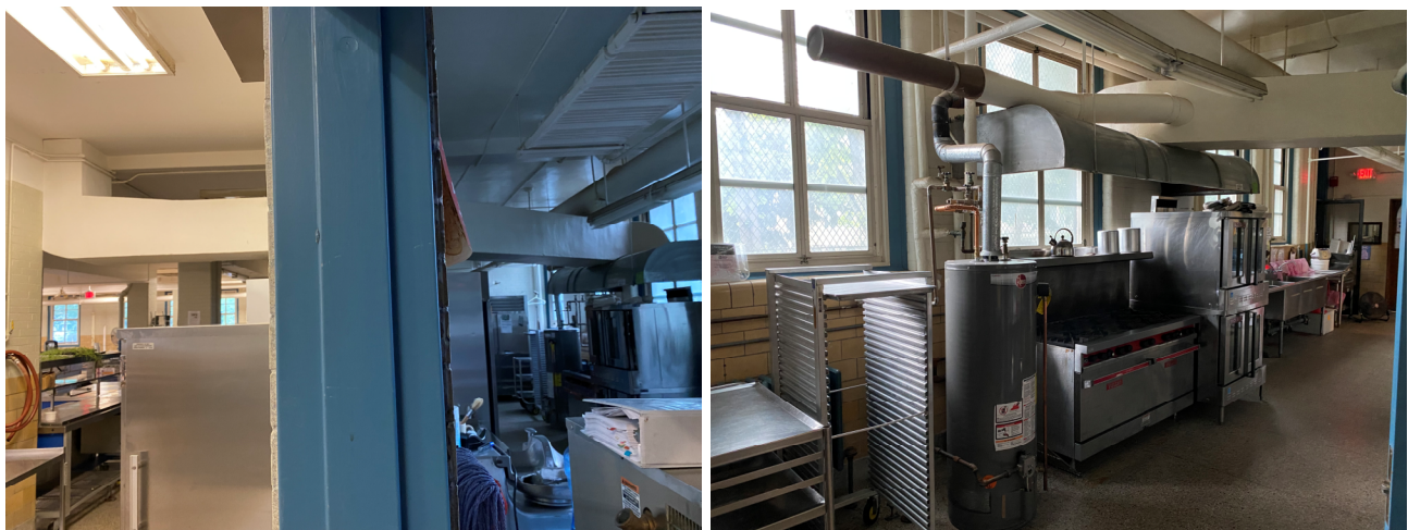
Photos 11 & 12: Existing Kitchen exhaust and DWH flue.
