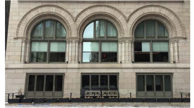
NEW WOOD FRAME AT OPERABLE AND FIXED WINDOWS - PAINT TO MATCH EXISTING
