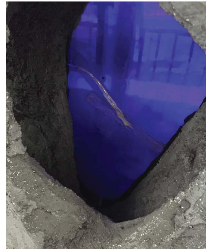
Detail at cracked glass
