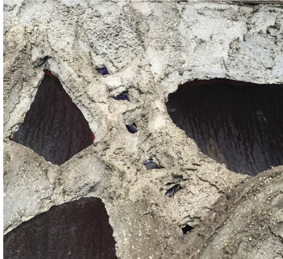
Detail view with exposed reinforcing
