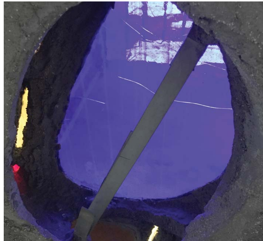
Detail at exposed metal support frame and cracked glass
