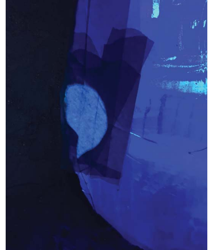
Detail at hole in glass patched with blue painter's tape
