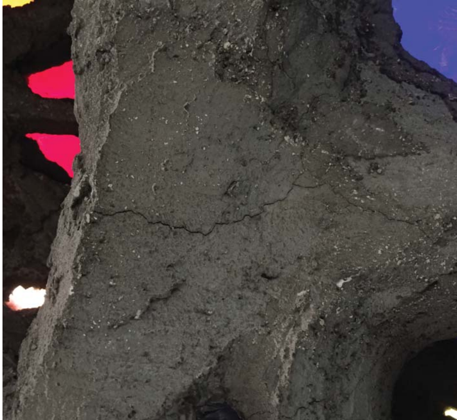
Detail at cracked cement
