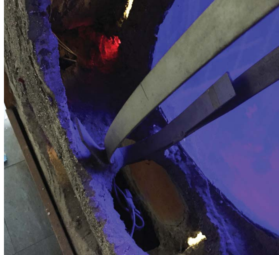
Detail of metal support frame and exposed wiring
