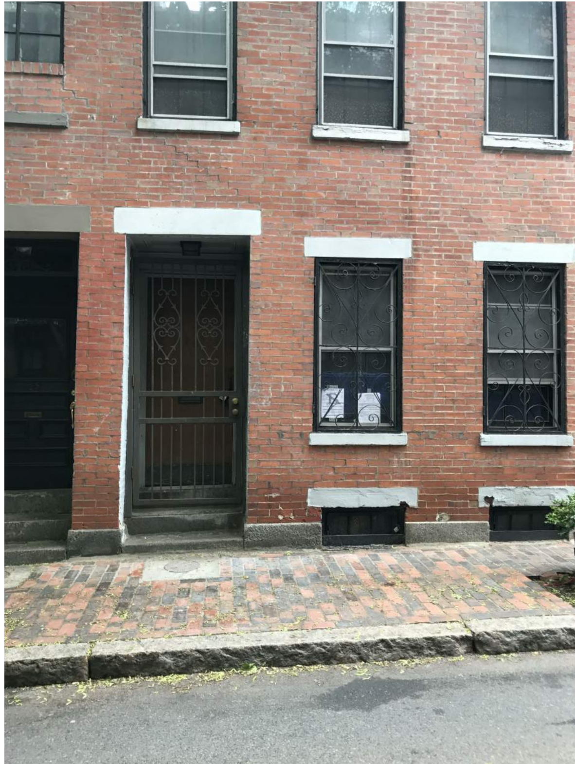
CURRENT CONDITIONS | 26 LAWRENCE METAL GATE AT FRONT DOOR AND METAL WINDOW GRILLES TO BE REMOVED
