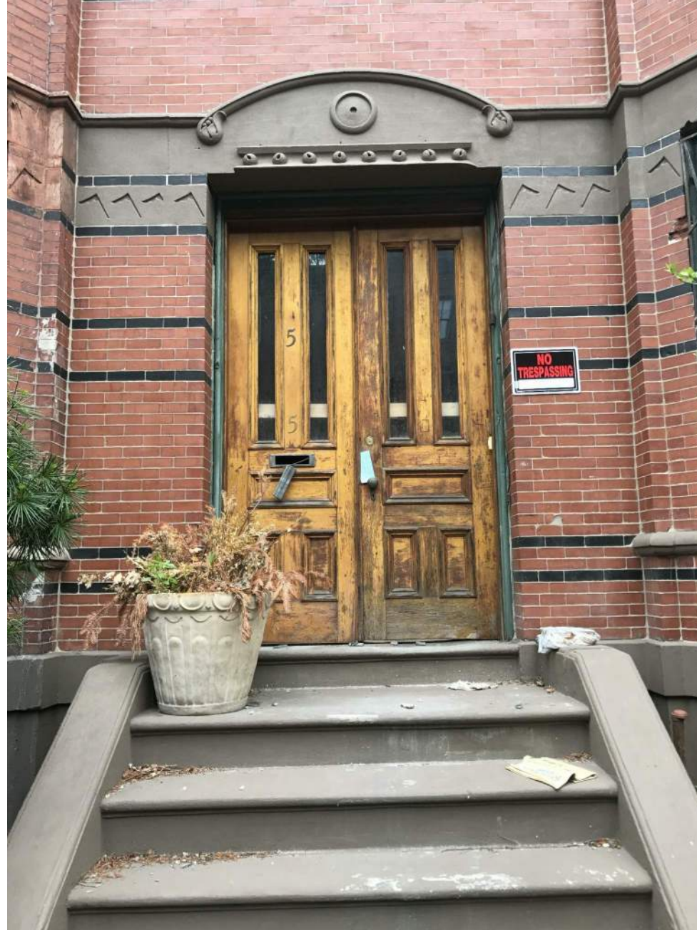
EXISTING DOOR TO BE REPAIRED AND RESTORED STOOP TO BE REPAIRED AND RESTORED
