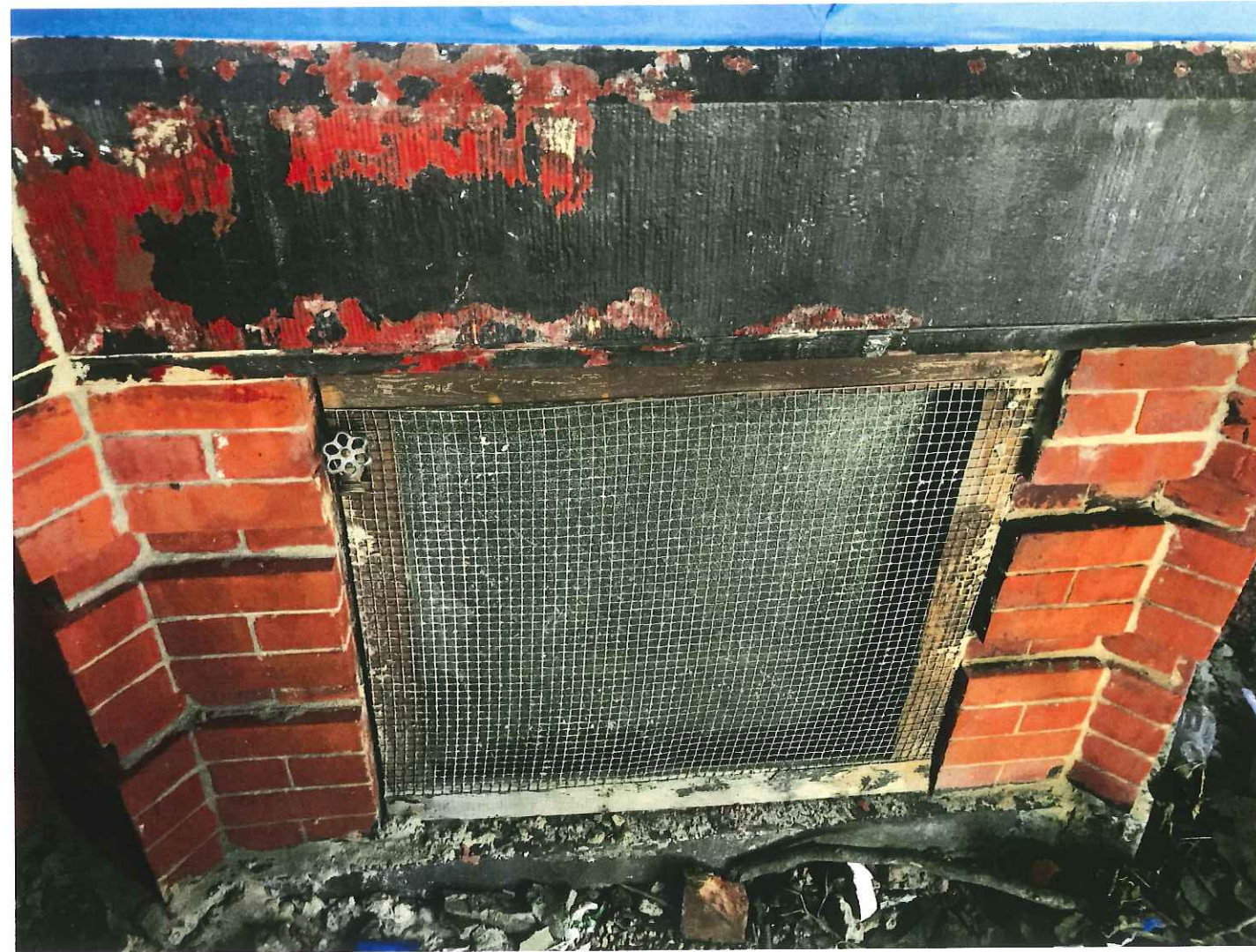
REMOVE METAL MESH SCREENS AT GARDEN LEVEL WINDOWS. REPAIR AND RESTORE MASONRY.
