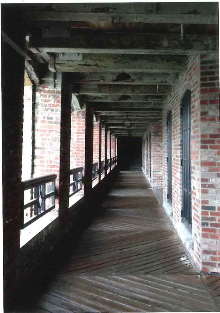
Harborwalk at lower level, 253 Summer Street (flooring is wet & appears darker in photo)
