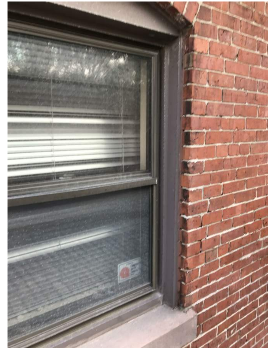
NON-HISTORIC REPLACEMENT WINDOWS AT ALLEY
