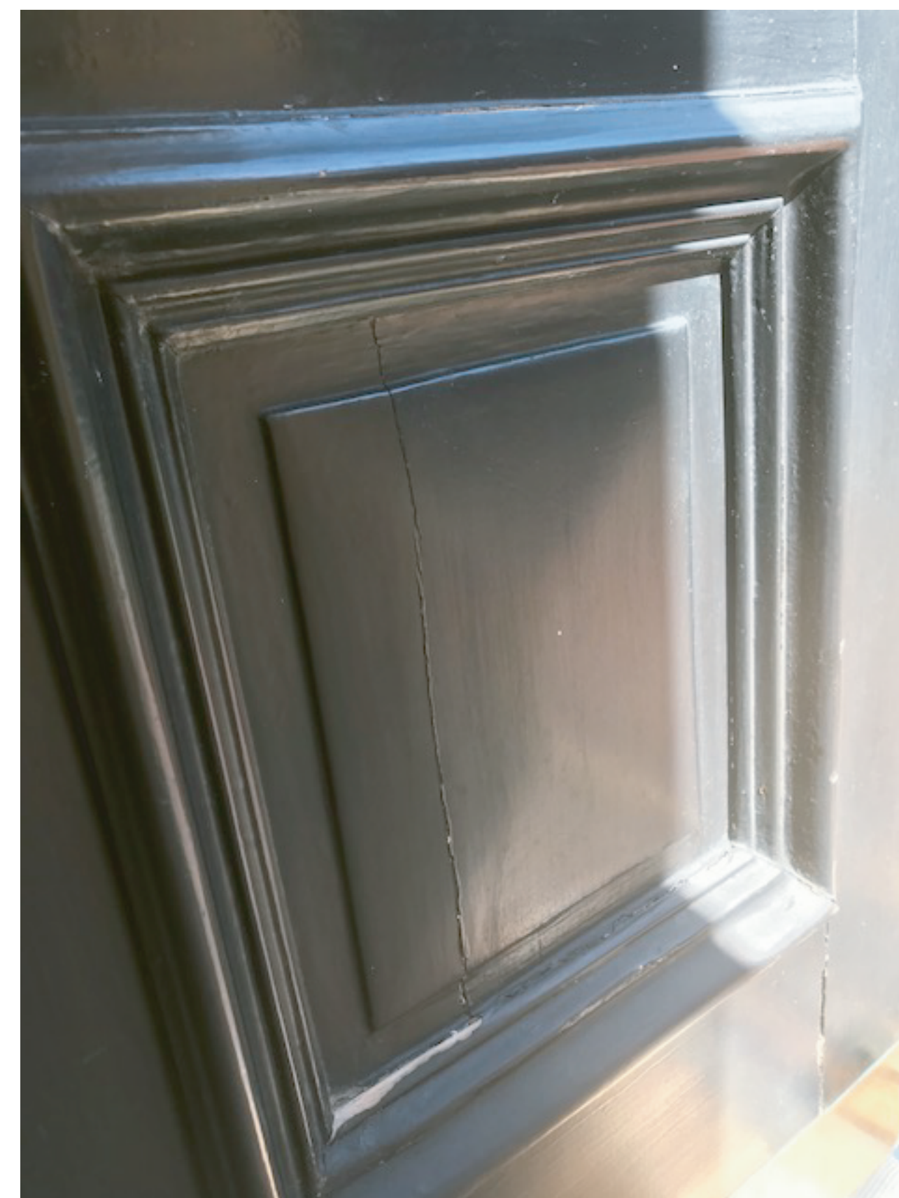
Cracked lower panel at exterior.
