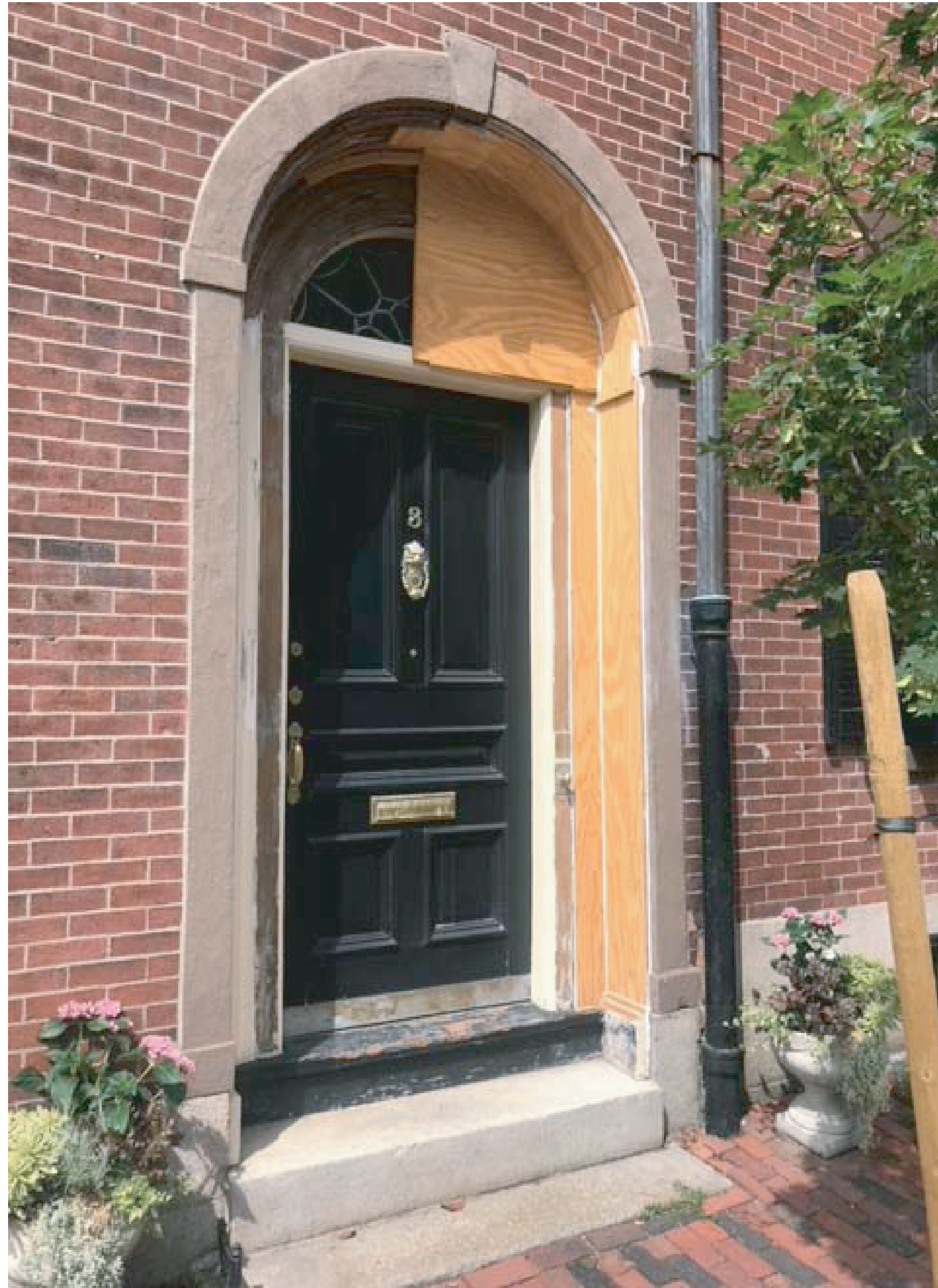
Front entry door for replacement. Existing door joints loose from swelling due to water damage. Select moulding was removed by fire dep't, to be replaced to match existing.
