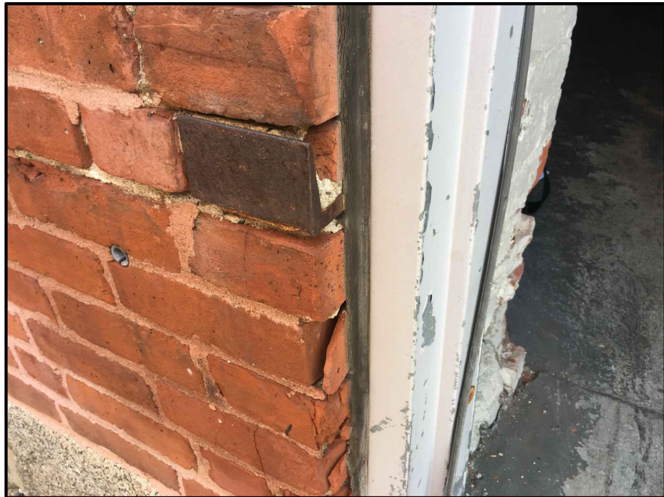
EMBEDDED FIRE SHUTTER HINGE CUT OFF
