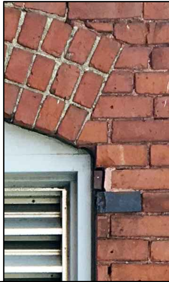
BRICK CUT OUT FROM BENEATH SEGMENTED ARCH
