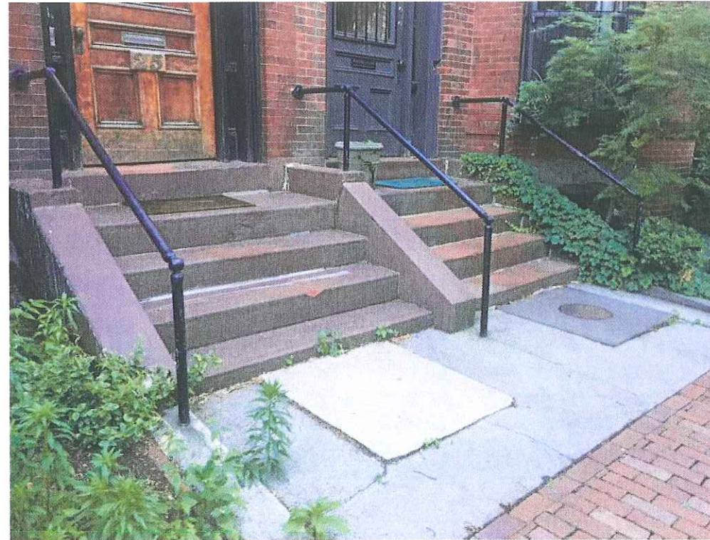
25-23 CUMBERLAND - PIPE RAIL AT STOOP; NO GARDEN RAILS
