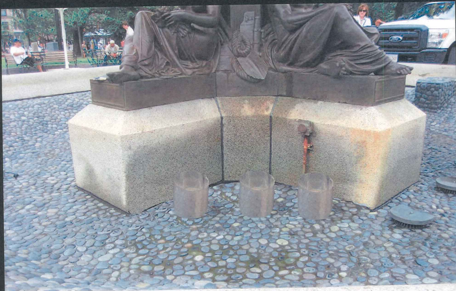
Proposed Design with Option Fixtures + shields sunk into floor of basin Fixtures rotated, shields identical orientation Pitch of top of shield reduced
