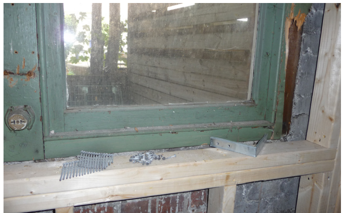
figure 8 | window A interior deterioration
