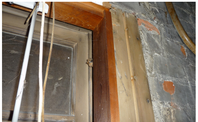
figure 12 | window B interior view Showing damaged sash cord
