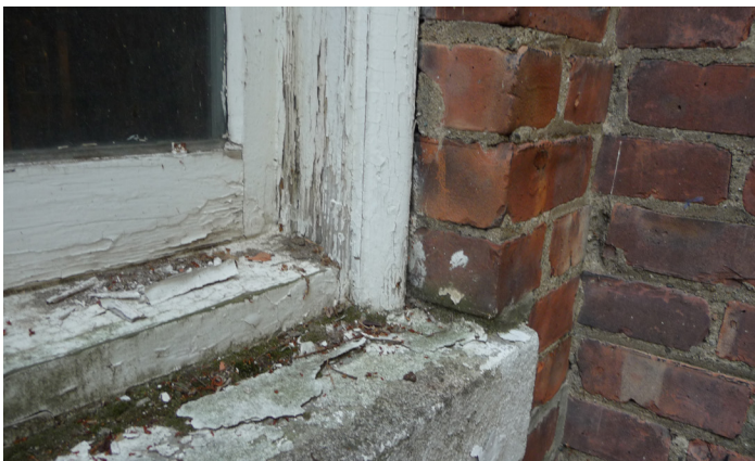
figure 7 | window A exterior deterioration
