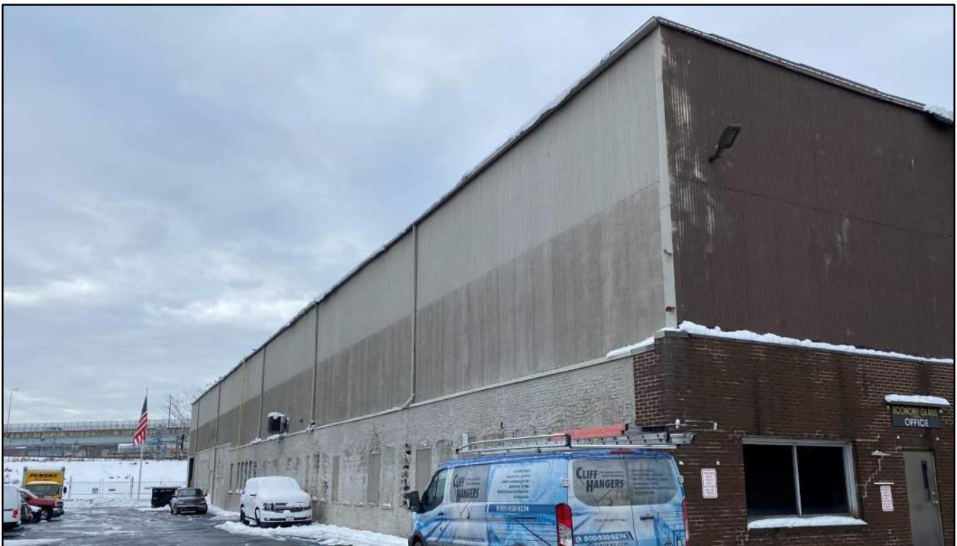
E6 – Southern Elevation View from Middle of Private Access Drive, Looking Northwest
