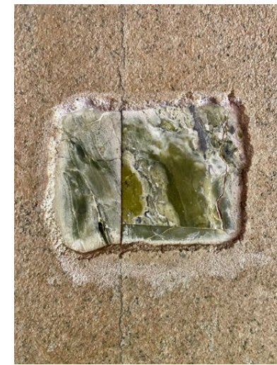
Green stone behind cementitious cladding at walls
