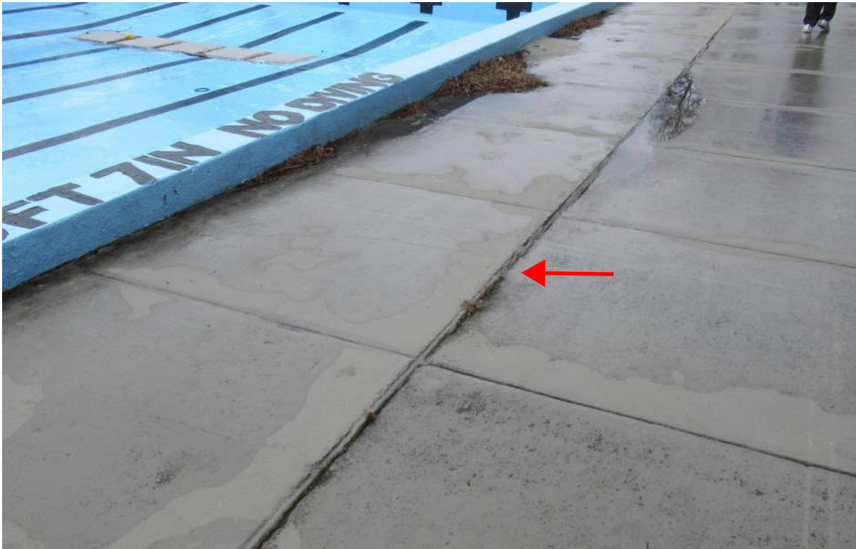
Photo 3: Irregular Apron Slab Surface - Trip Hazard
