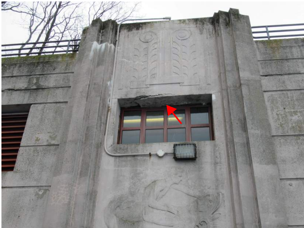
Photo 2: Soffit Concrete Spall, North Wall of Bathhouse
