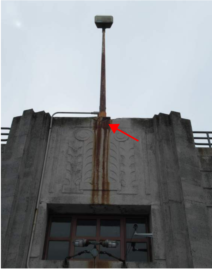
Photo 1: Base of Flagpole Concrete Spall, North Wall of Bathhouse
