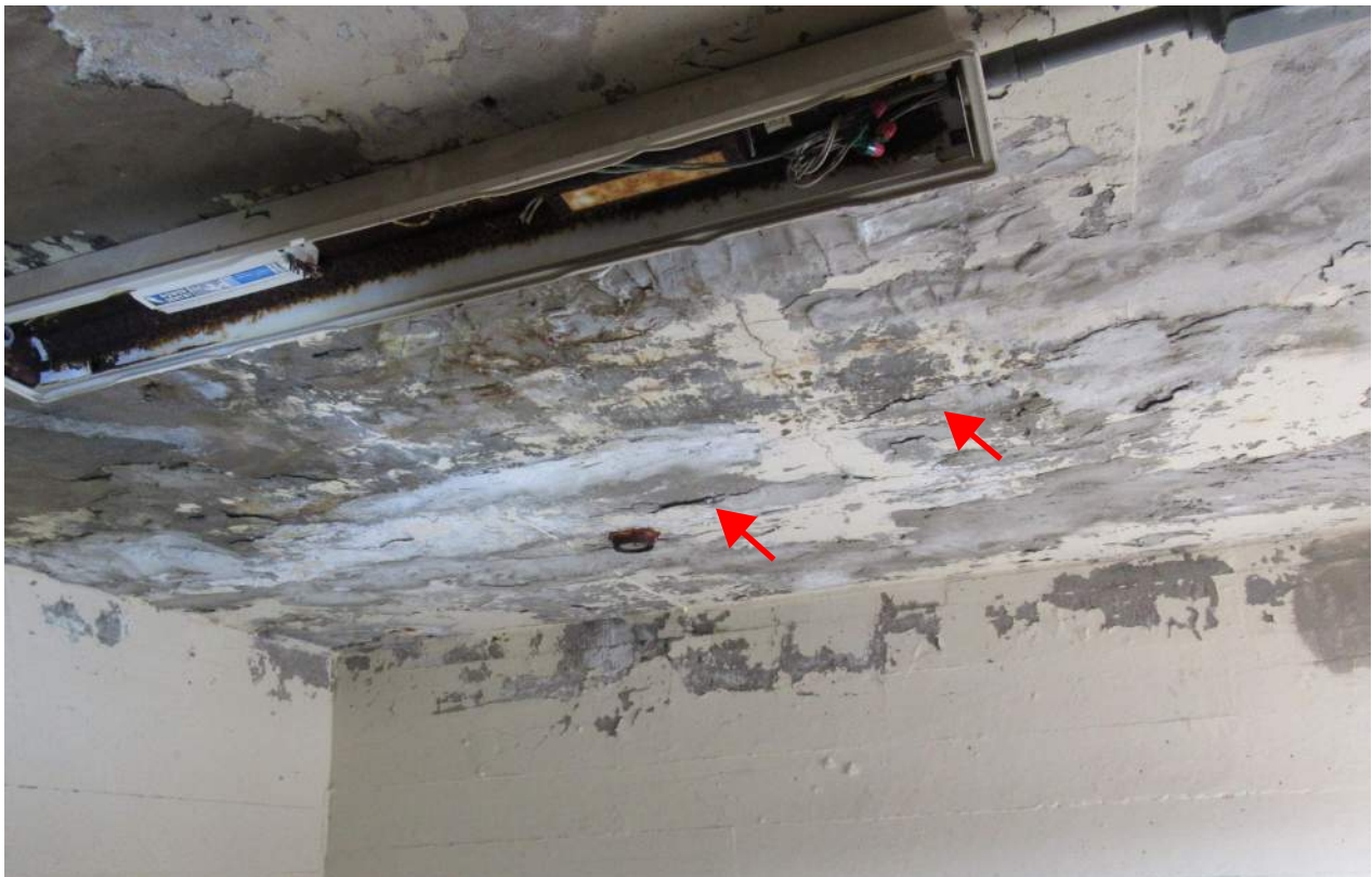
Photo 4: Concrete Spalling, Ceiling of Filter Room Headhouse
