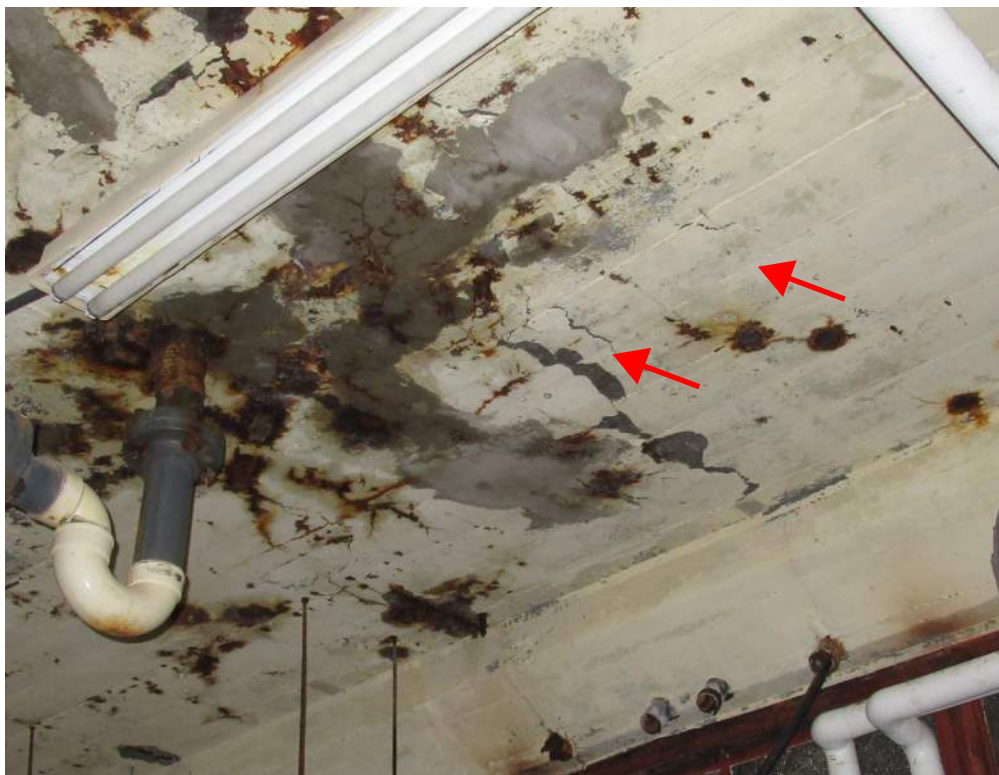
Photo 6: Bathhouse Ceiling Concrete Spalling
