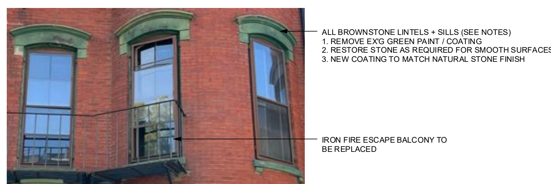
PHOTO 2.1 - REPLACE WINDOW (REFER DETAIL 5) RETAIN/ REPAIR LINTEL AND SILL, PAINT FINISHED (SEE NOTES)
