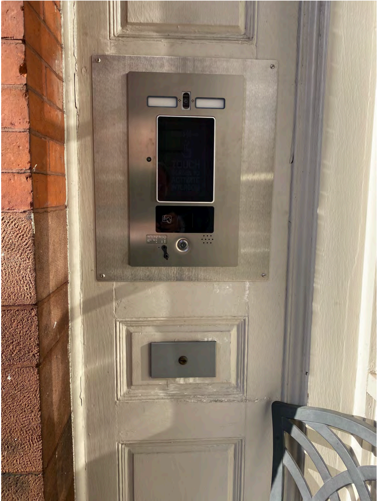
Existing Butterfly MX Intercom System to Left of Entrance in Door Surround
