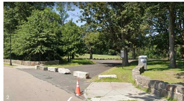
2 The historic carriage entrance with granite boulders used to block car access.
