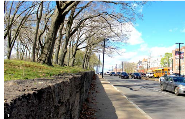
The puddingstone perimeter wall condition.
