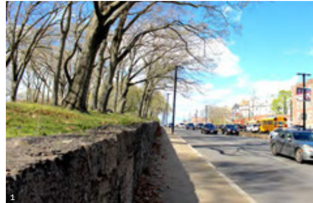
The puddingstone perimeter wall condition.
