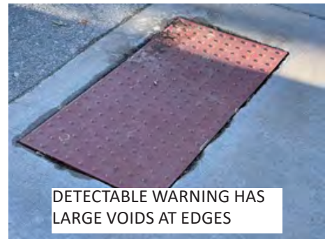
EDGE OF GRANITE PAVING IS A TRIPPING HAZARD
