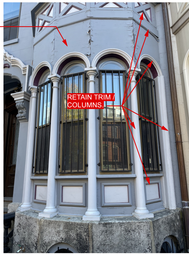
WOOD BAY CLOSE-UP
