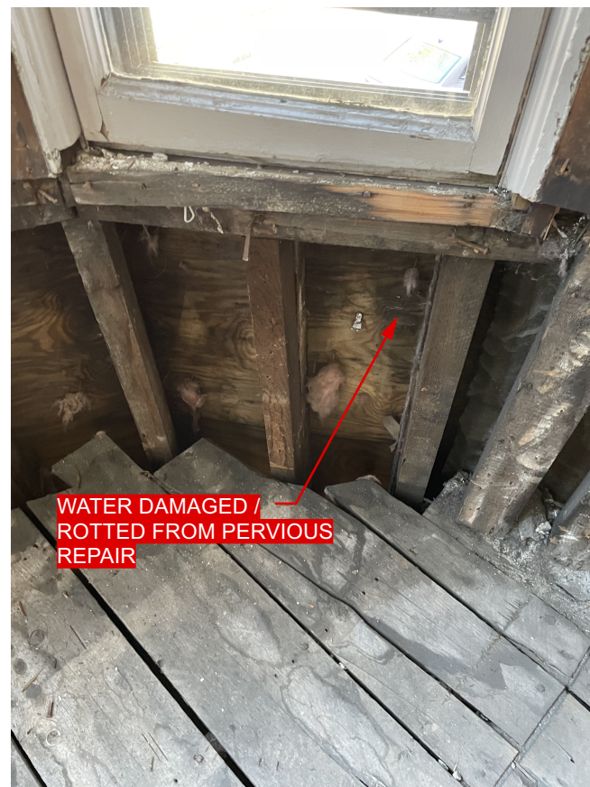
WOOD BAY ROT / WATER DAMAGE
