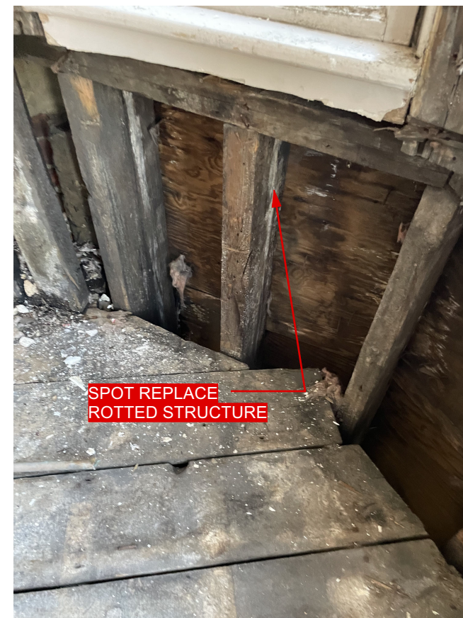
WOOD BAY ROT / WATER DAMAGE
