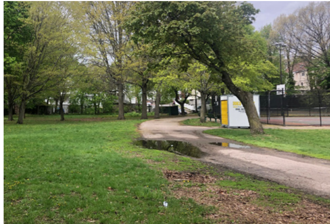
Settling Paths & Drainage Issues
