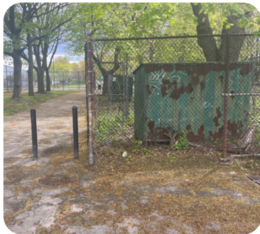
Utility Cabinets (Poor Condition)
