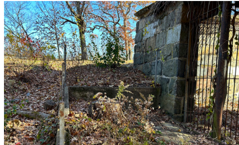
Retaining wall, fall hazard
