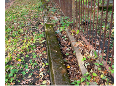
Settling curbing, trip hazard
