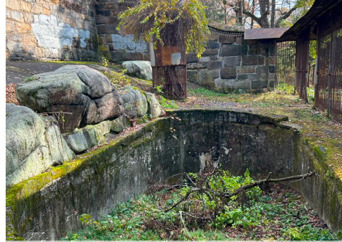
Pool - fall hazard, organic matter build up
