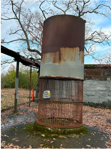
Tree cage instability Recommendation: Secure structure and close open access panel
