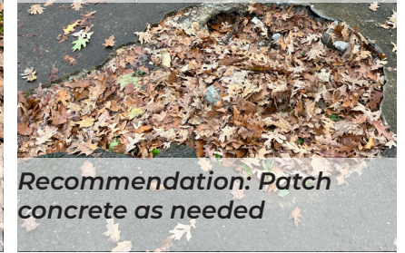
Concrete pavement void, trip hazard
