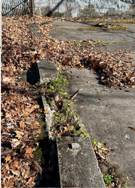
Curb dividing cages, trip hazard
