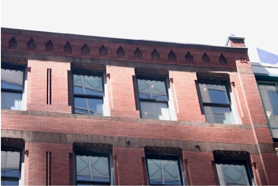
Figure 14. Upper levels and roof edge, 115-119 Pearl St. façade. Photograph by Wendy Frontiero, June 2023.
