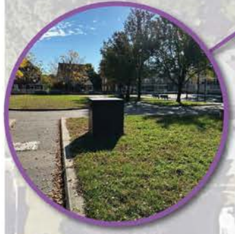
- UTILITIES BOX IN PROMINENT AREA
