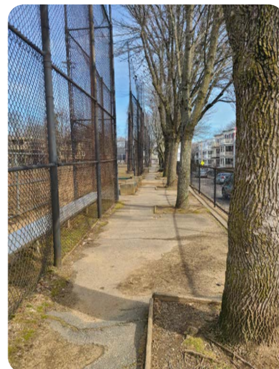
Edges of Tree Wells Have Been Heaved by Tree Roots
