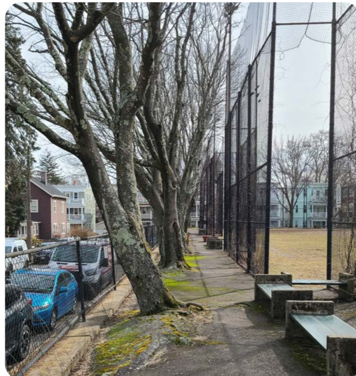
Path Heaved by Tree Roots Creating an Uneven Walking Surface
