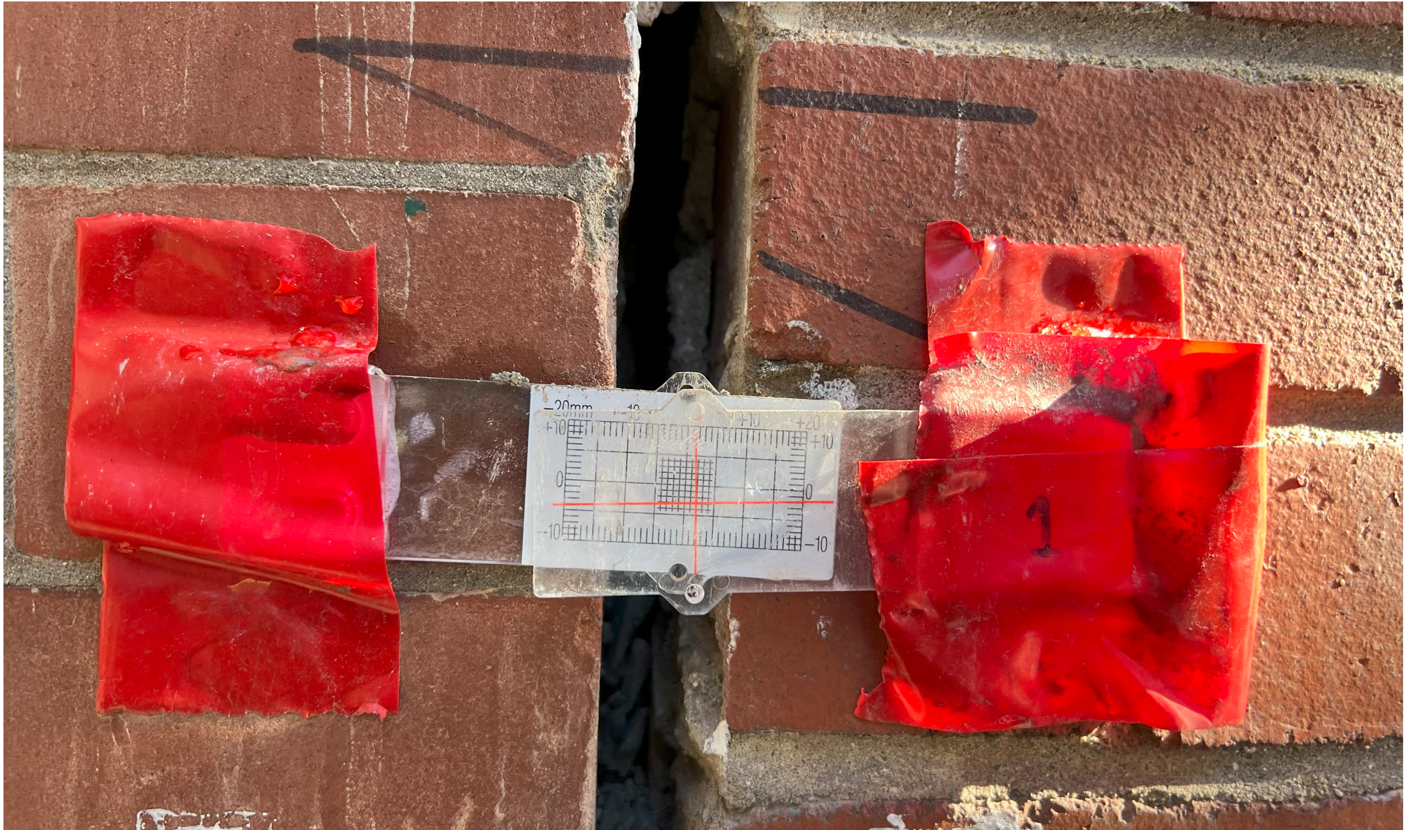
STRUCTURE SETTLEMENT MONITORING DEVICE STRADDLES OVER 151 CHARLES STREET, AND 147 CHARLES STREET
