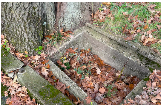
Several tripping hazards
