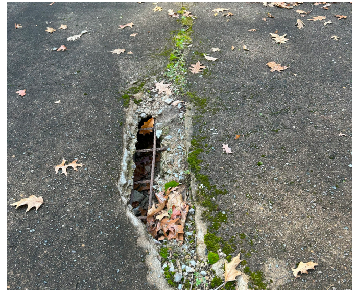
Areas of failing concrete; sink holes
