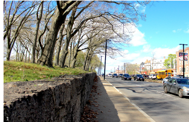
The puddingstone perimeter wall condition.
