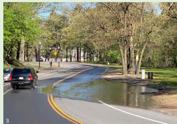
Flooding on Circuit Drive after a rain storm.
