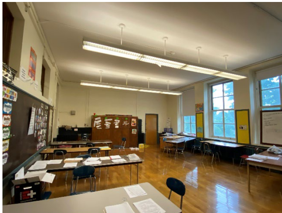
Classroom Pendant 1'x4' - 2 lamp fixtures
