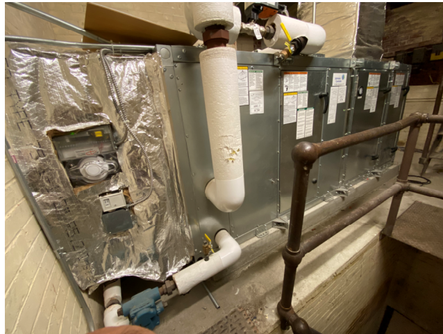
Photos 13: Existing AHU serving the Auditorium.
