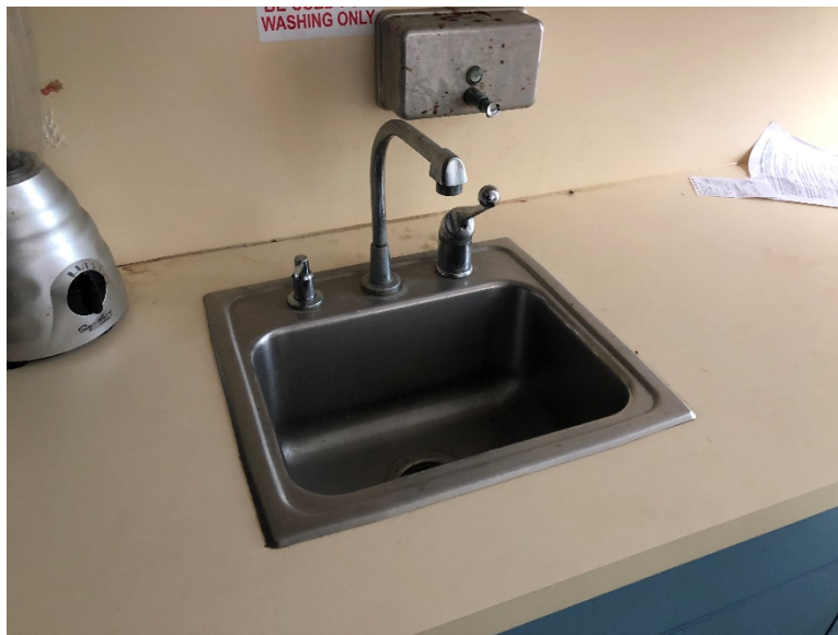
Photo 13: Typical General Use Sink
