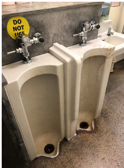
Photo 10: Floor Mounted Urinals
