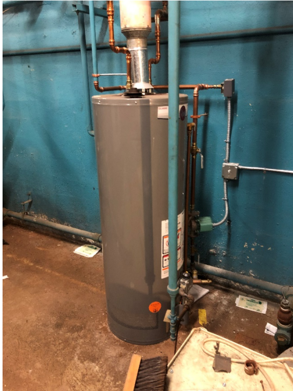
Photo 3: Gas Fired Water Heater
