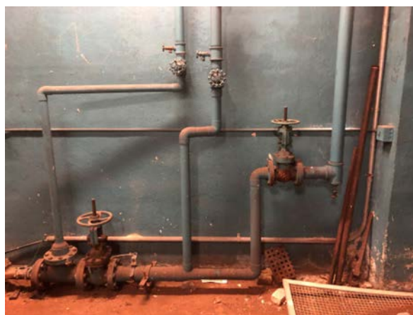
Photos 1 & 2: Domestic Water Service
