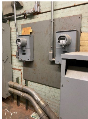
Main Disconnect Switch & Meters
