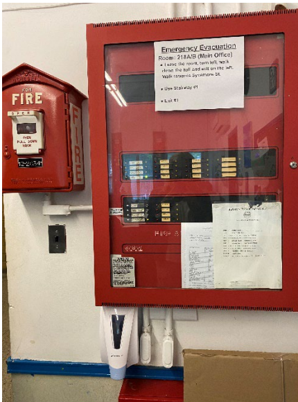
Fire Alarm Control Panel and Master Box
