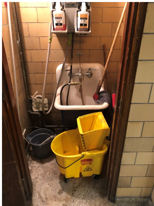
Photo 12: Cast Iron Mop Sink with Detergent Dispenser
