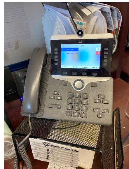
New Telephone System
