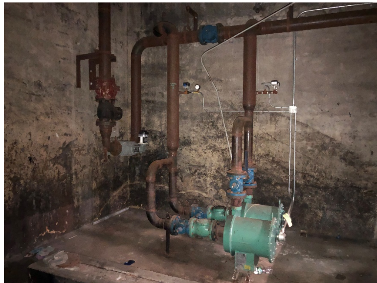
Photo 5: Gas Pressure Booster System
