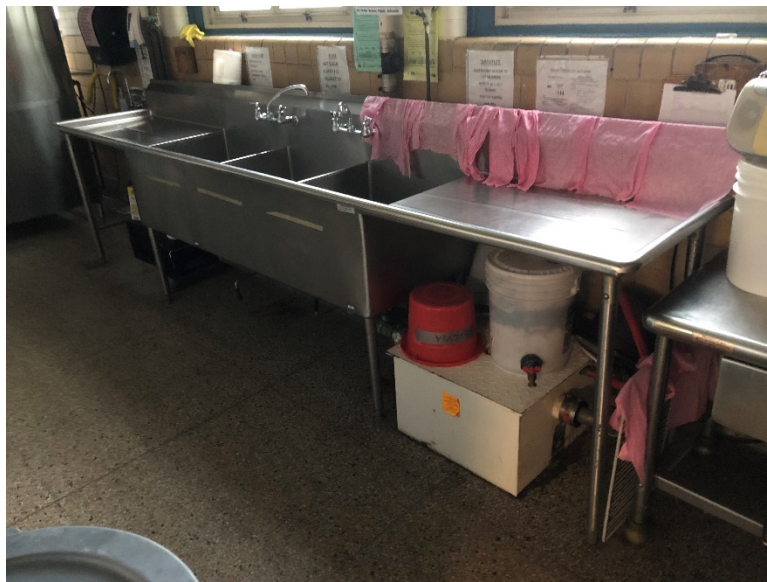
Photo 16: Scullery Sink & Grease Interceptor
