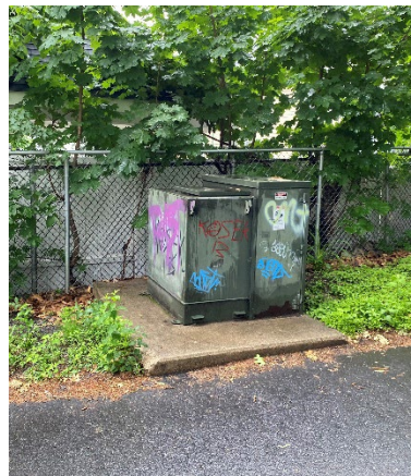
Utility Company Pad-mount Transformer
