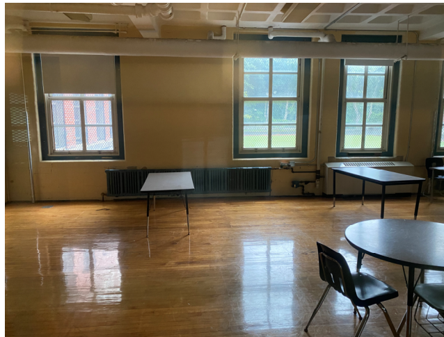
Photos 10: Typical classroom radiator and unit ventilator.
