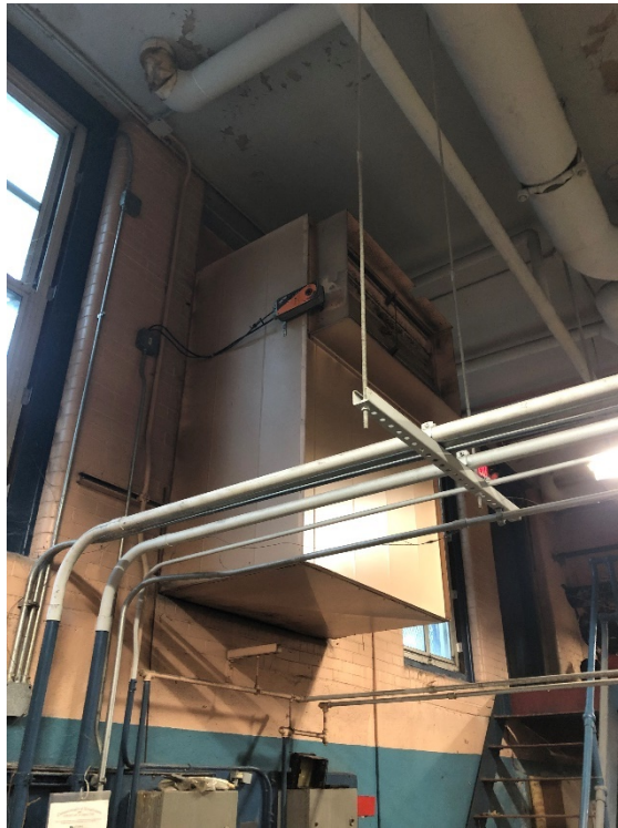
Photo 6: Combustion Air Duct
