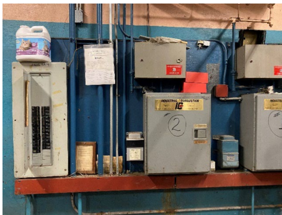
Feeder Circuit Breaker Panels
