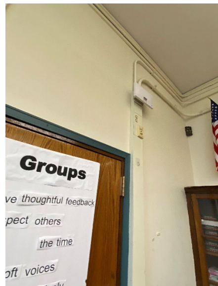
Wireless Access Point Devices
