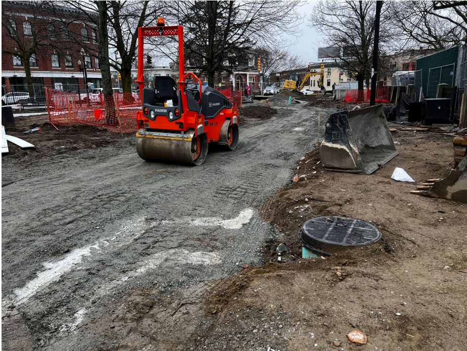
The paving base course below the new concrete walkways has been installed.
