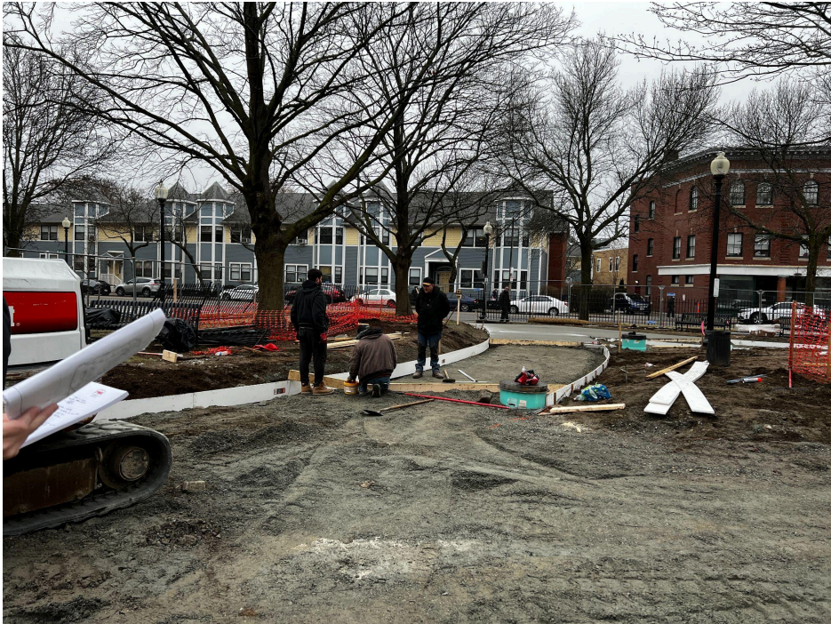
The contractors are carefully laying out expansion joints for the concrete pours.
