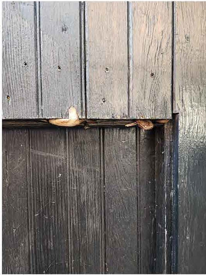
Rot & Fungus @ Header
