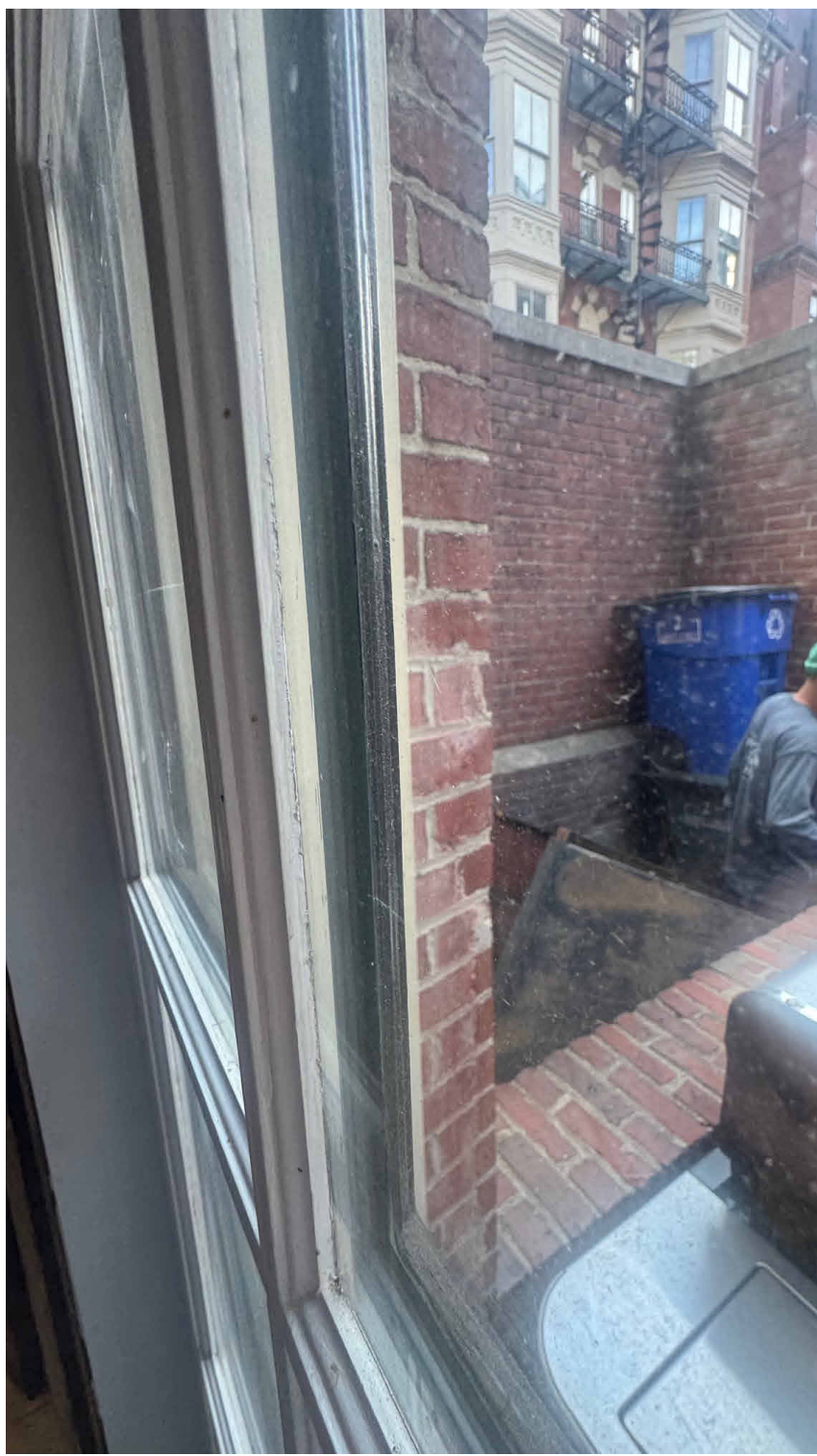
EXISTING NON-HISTORIC WINDOW CLOSE UP SHOWING EXISTING SIMULATED MUNTINS
