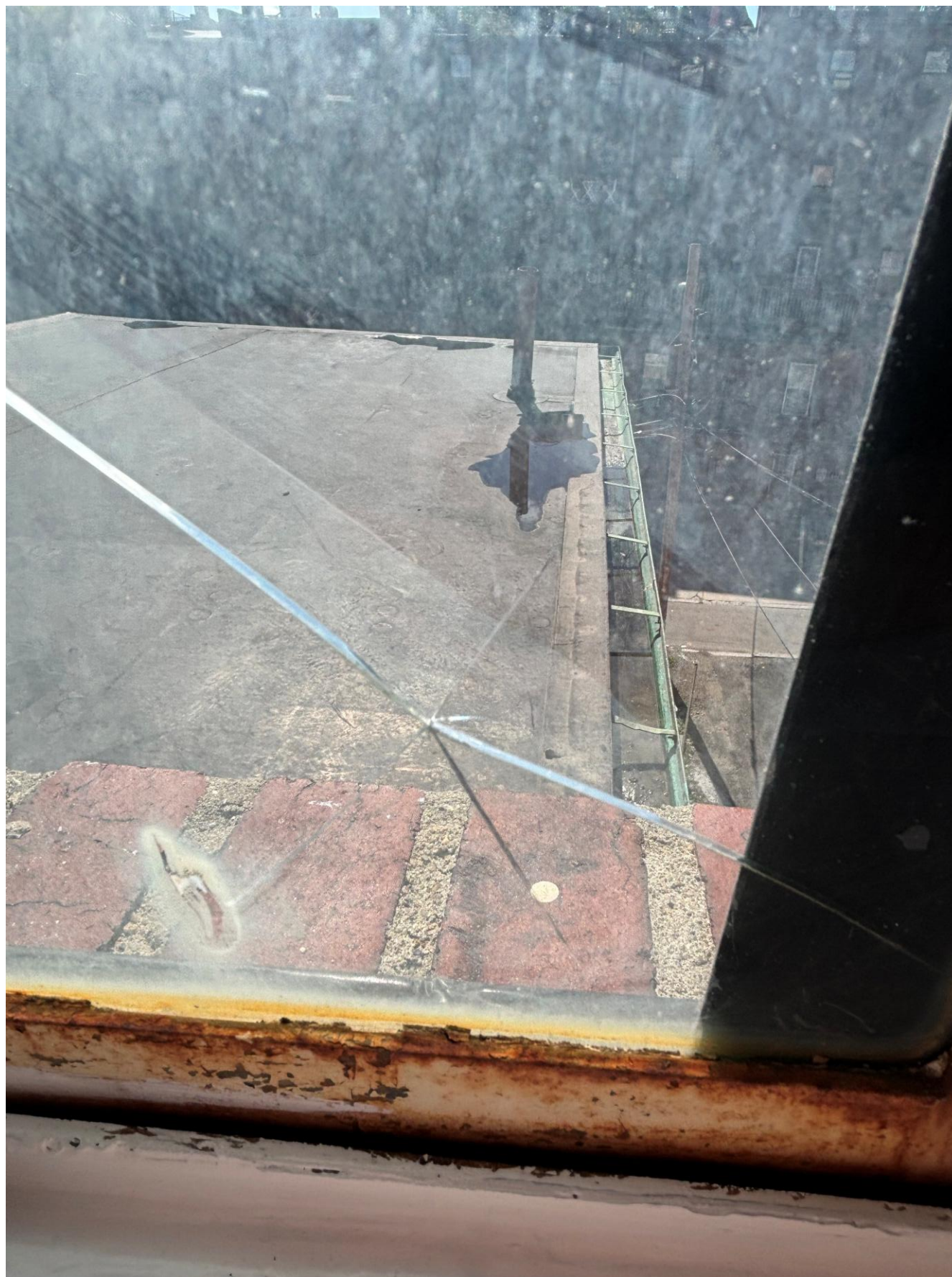
BROKEN PANE ON WINDOW 1
