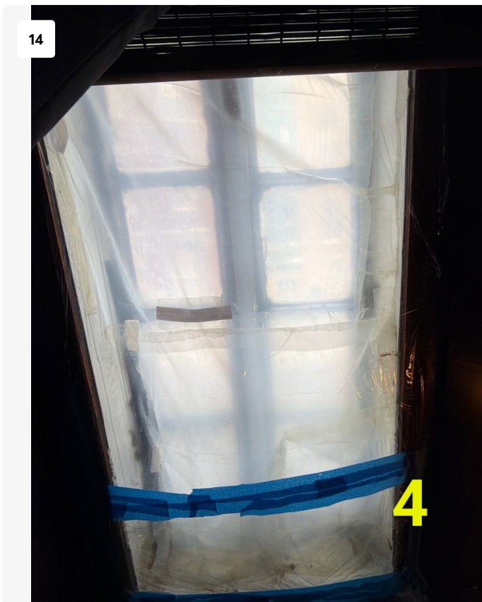
Current window 4 interior. Window does not close so resident has sealed off window.
