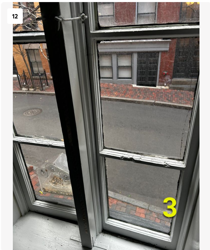
Deteriorated muntin bars
