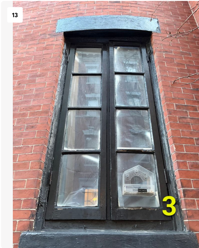
Deteriorated window sash & frame
