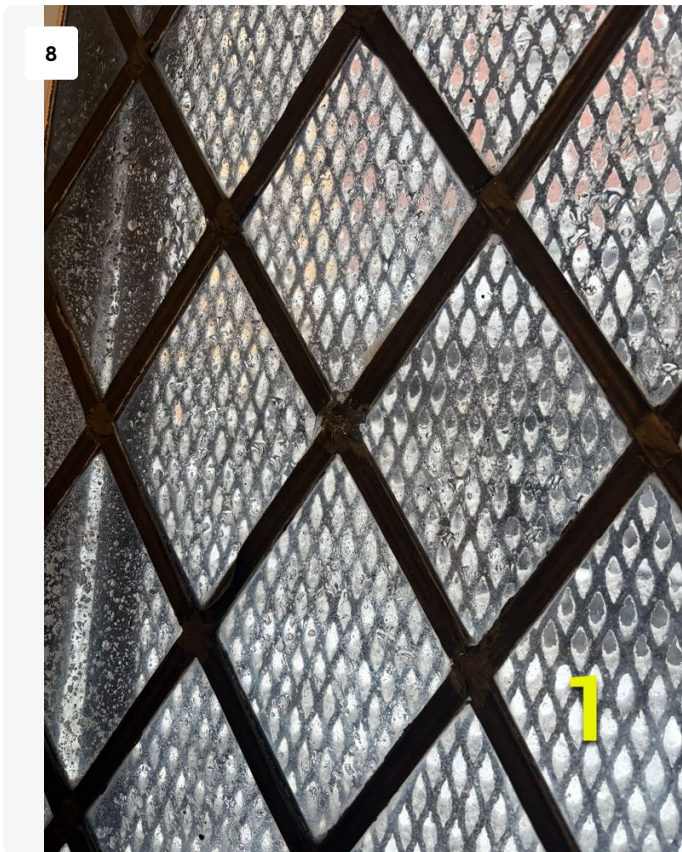
Glass repaired with glue in multiple locations
