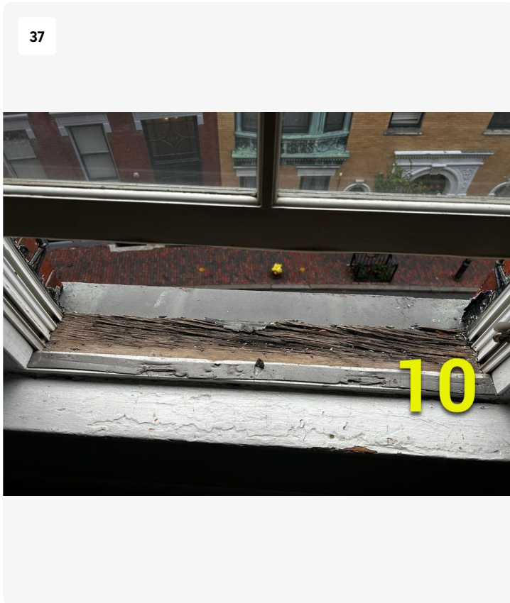
Deteriorated sill as is consistent across all windows
