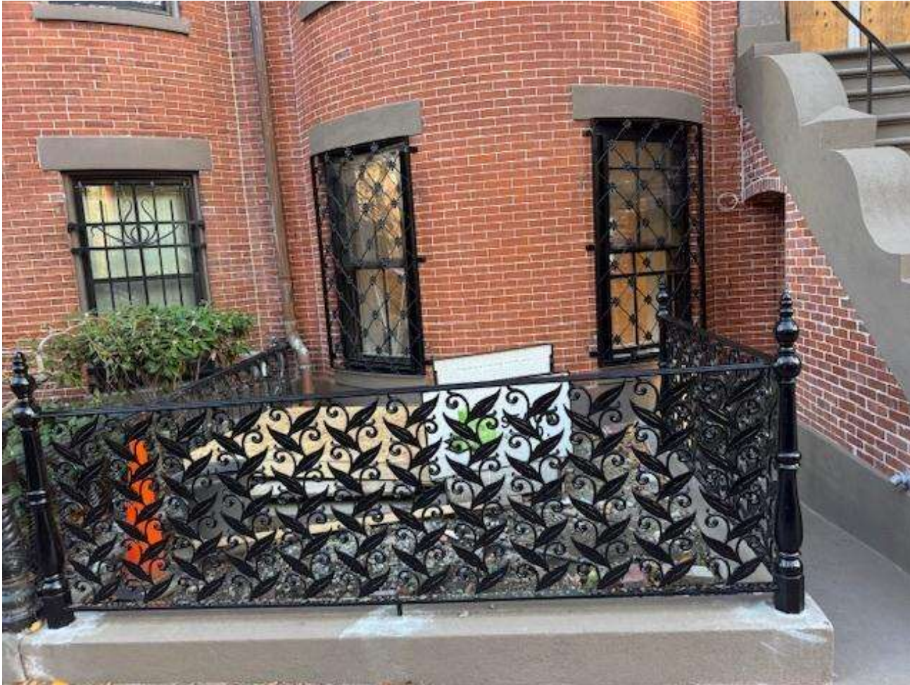
Installed unapproved garden fence
