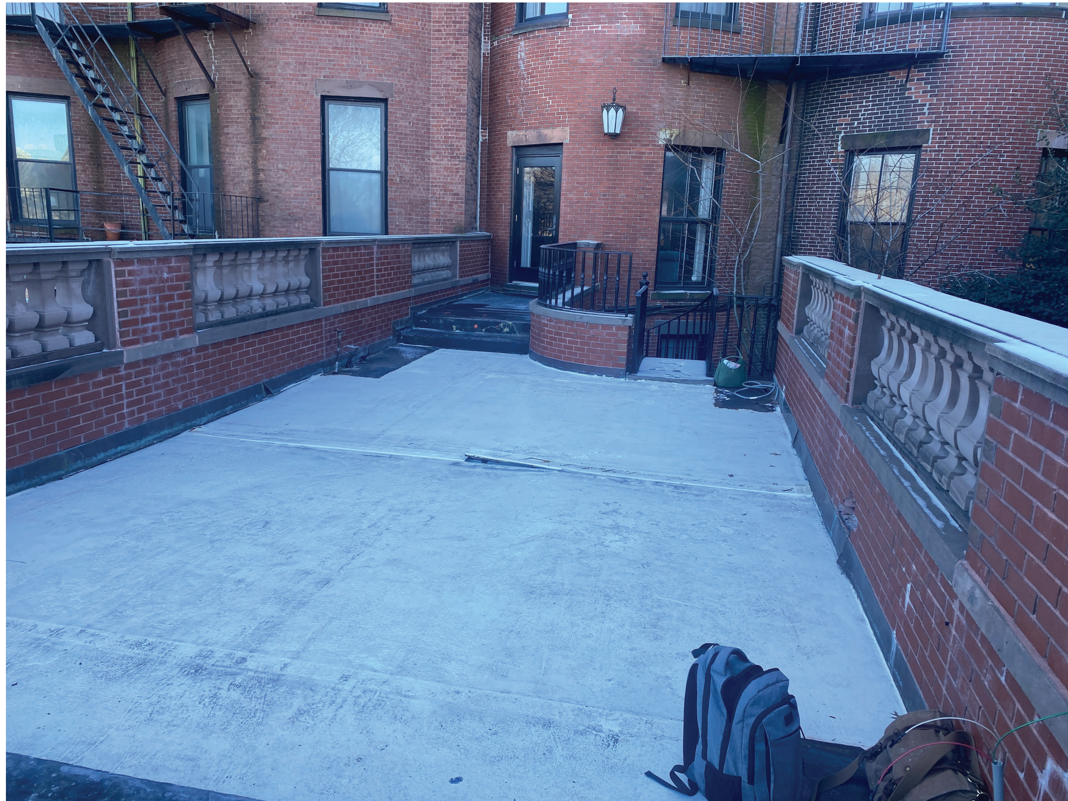
January 2026 - removed pavers showing failing membrane roofing
