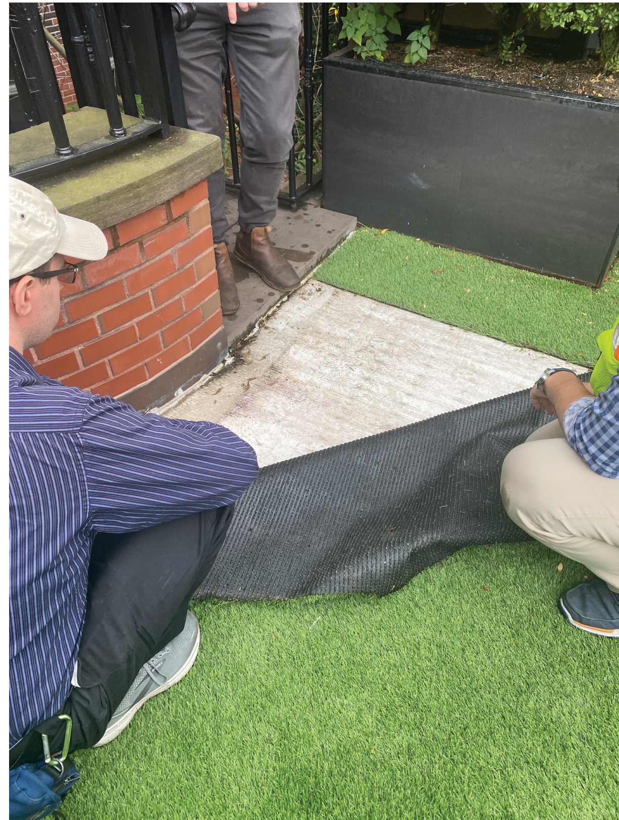
September 2025 - failing membrane roofing below outdoor carpet and stone pavers
