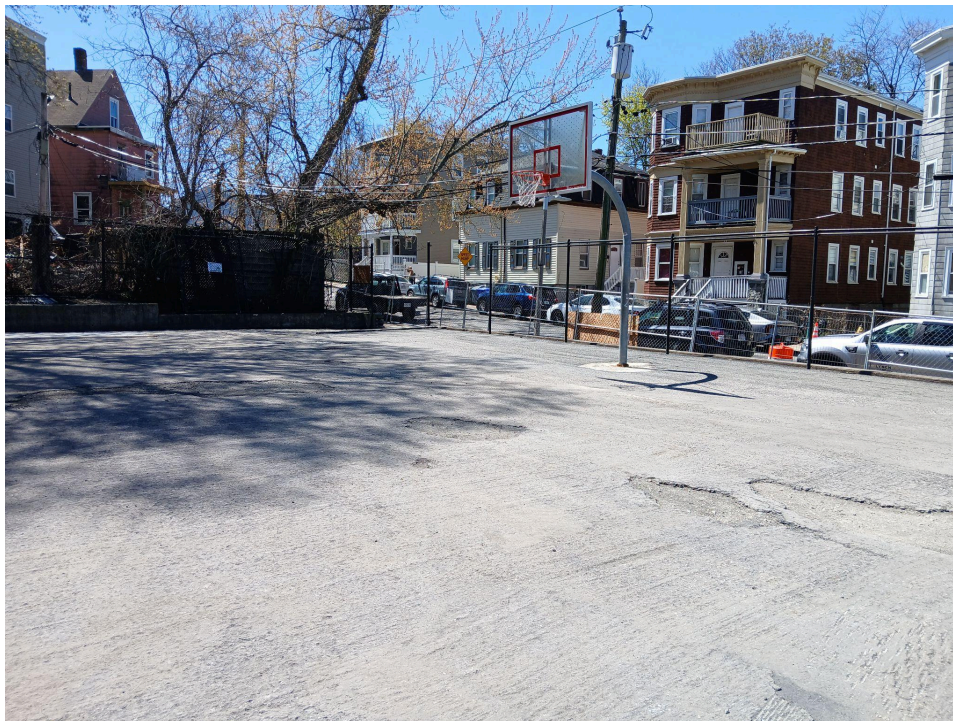
Ripley Playground in Dorchester: basketball court top surface was removed and site prepped for new course of asphalt.
