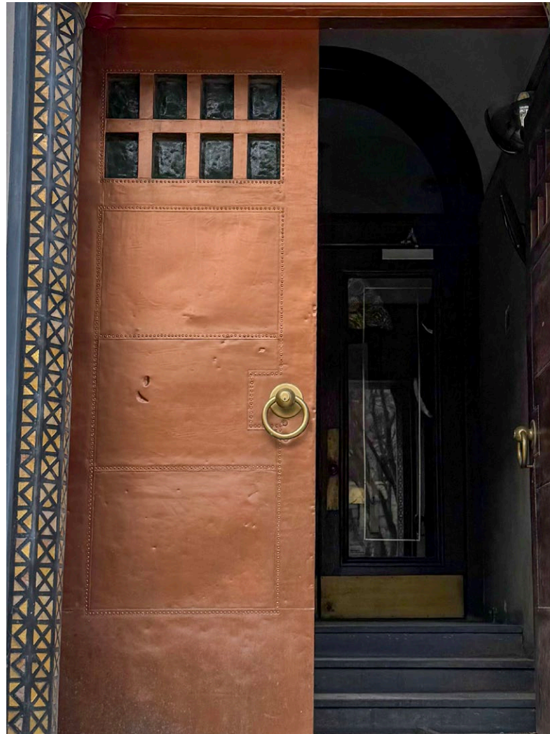
Copper clad entry door, dents cannot be repaired, copper is not punctured
