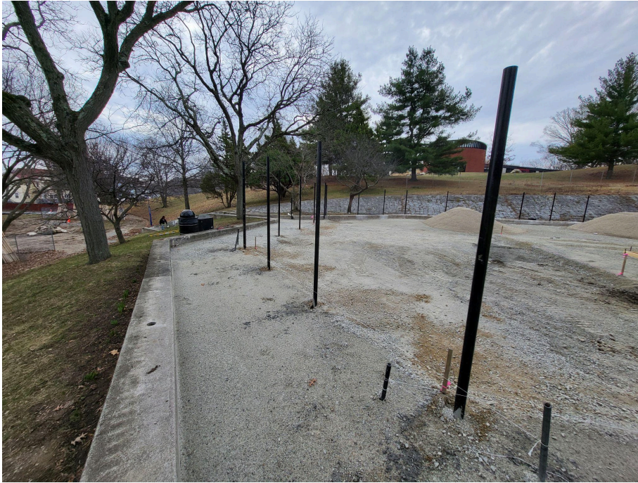
The dog park fencing and paving subbase material in the process of being installed.
