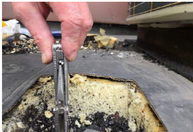
Test cut found 3.25" flat polyiso over two layers of built-up roofing, over wood deck. All layers are to be removed down to the wood plank decking, then a new insulated modified bitumen roof system is to be installed at both the main roof and the north penthouse roof.
