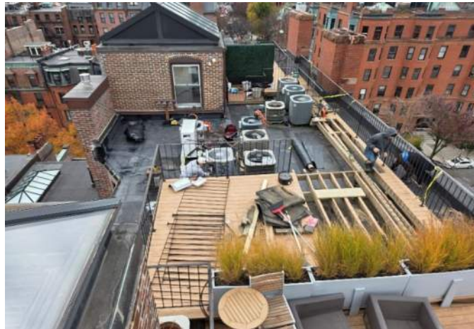
View of Main Roof, taken from the Penthouse Roof, looking south. Main roof and north penthouse roof are to be removed and replaced. No work is to be done at the south penthouse roof. Roof decks are to be removed and replaced with pedestal paver patios.
