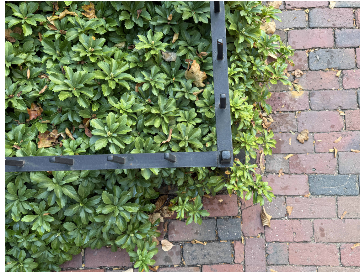
South Fence Corner to be Replaced
