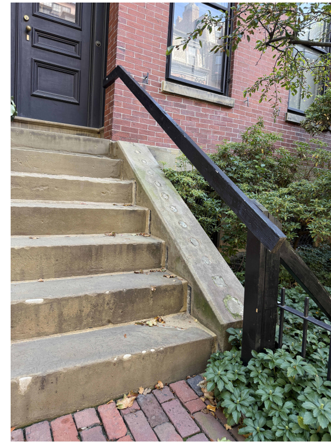
South Handrail to be Replaced
