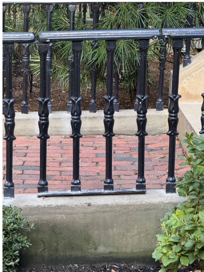
Neighboring Gate to be Model for New Gate
