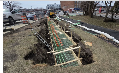
Deployable Flood Walls
