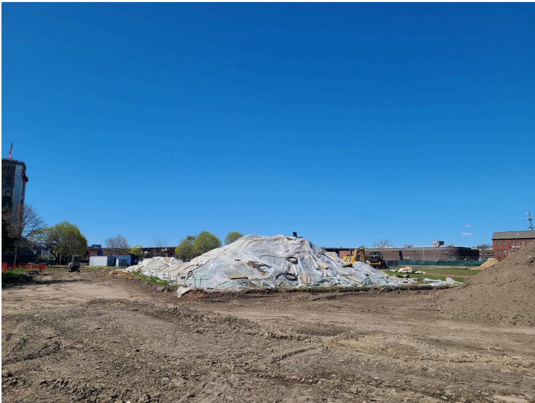
One of the mountains of excavated soil, protected with tarps to prevent dust.
