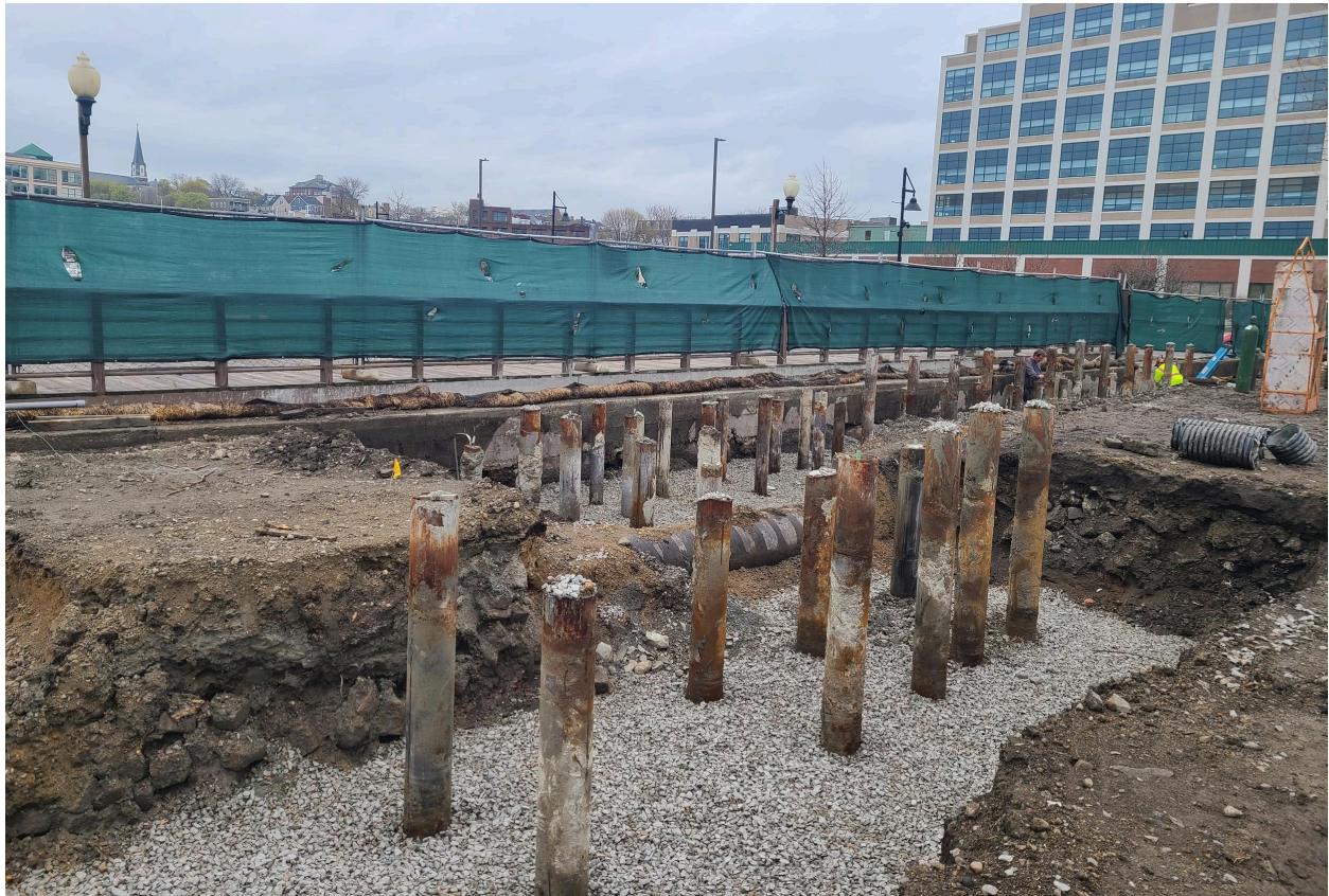
Tops of the piles that were installed in Phase 1 need to be cut, and rebar in the center will be exposed, so the pile cap can be attached. This photo is adjacent to the fishing pier, looking back at Schrafft's.
