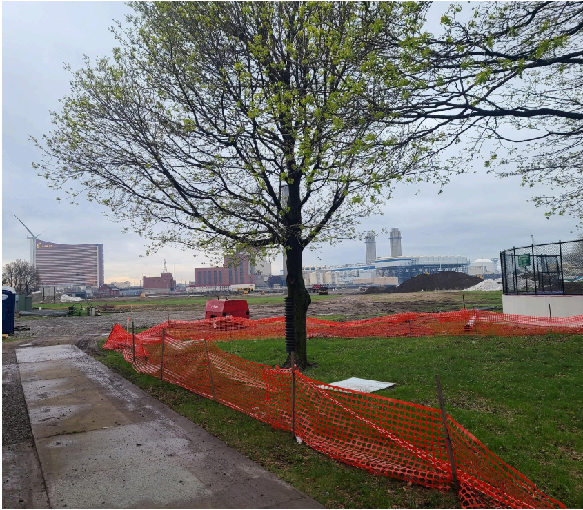
Orange construction fence marks the Critical Root Zone of trees that will be preserved and protected during construction. We require tree protection to be in place before the construction begins.
