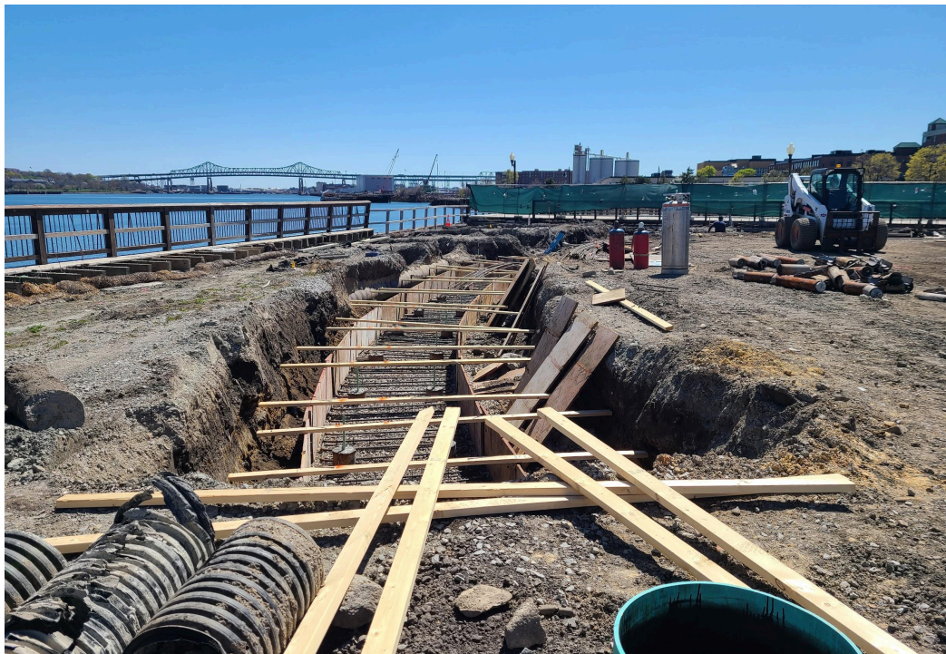
In the corner of the site near Schrafft's the seawall curves, which you can see here. They have rebar set up and plywood forms, preparing for the concrete base.
