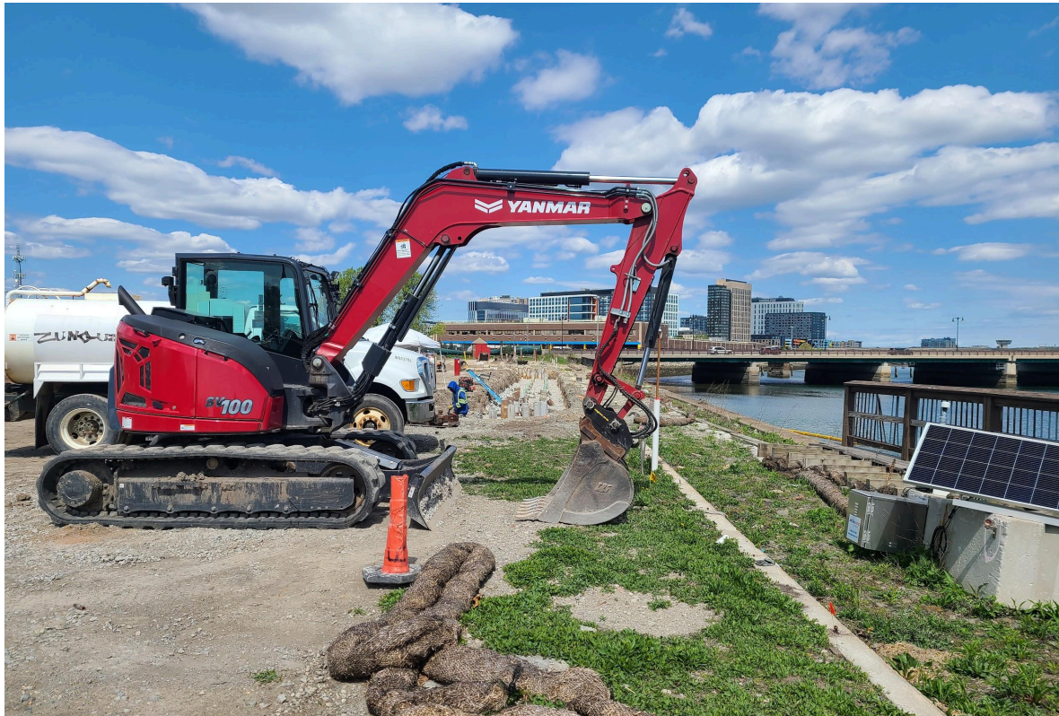
Looking towards the Alford Street bridge, the tops of the piles are visible in the area of the berm where the playground will go. The wall attached to these piles will be formed with rebar, and poured concrete next, and should be visible in early June.
