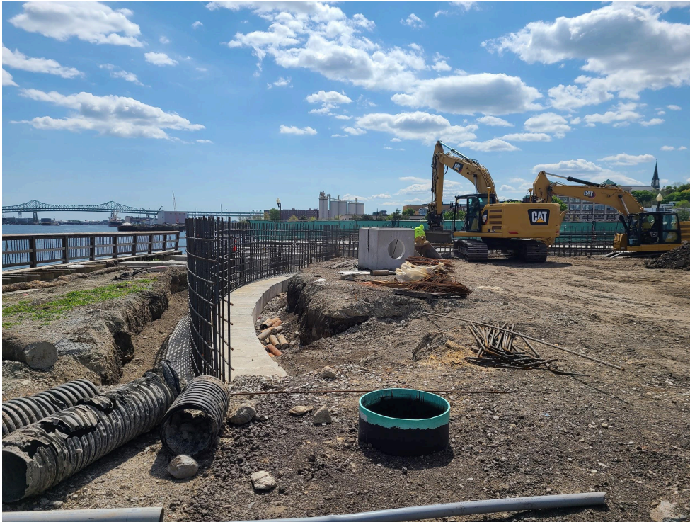
By the corner of the park with Schrafft's, the curved base of the berm will be supported by this wall, which has rebar almost ready for the concrete pour.
