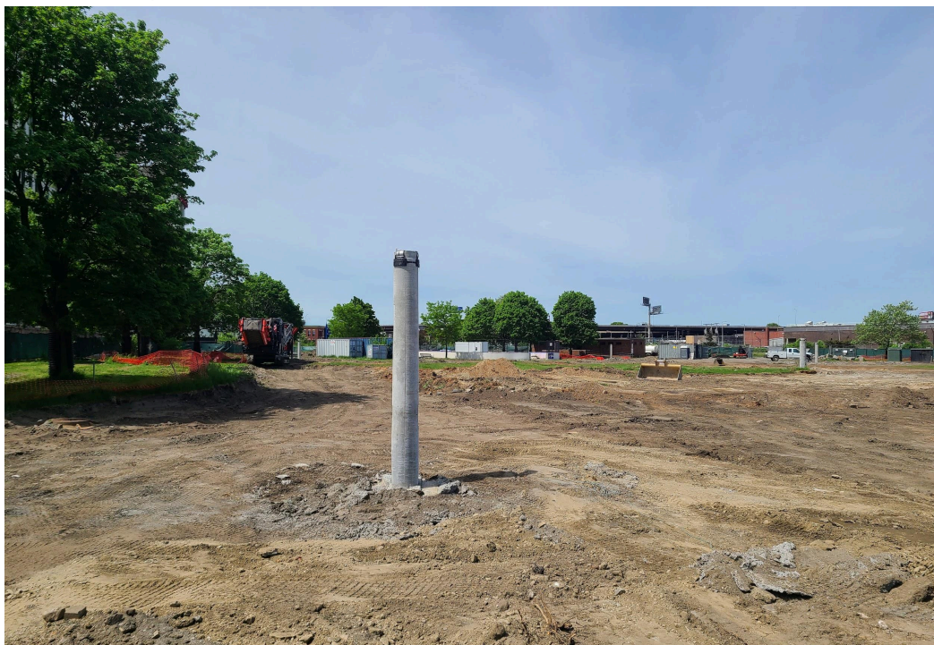
A concrete light pole base, waiting for the light to be installed.
