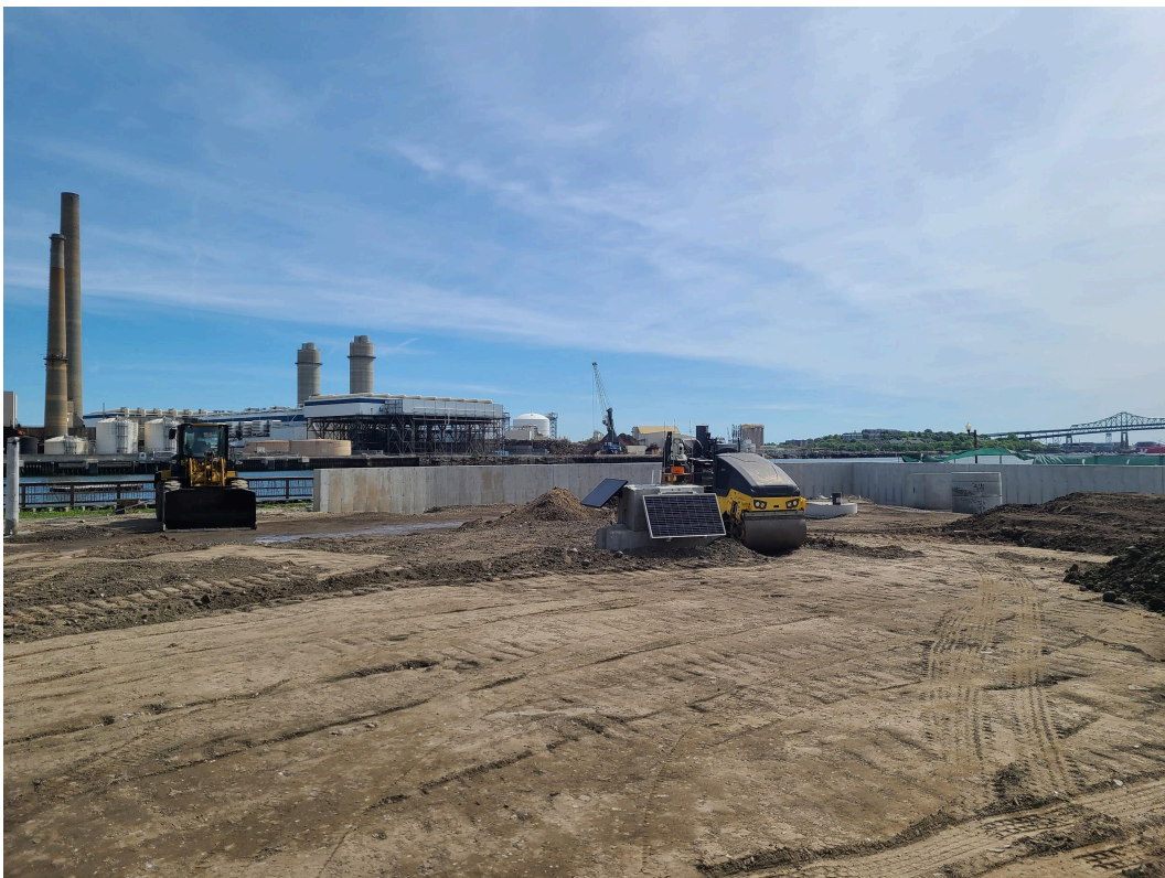
The same area - shown from a different angle - with the concrete wall poured.
