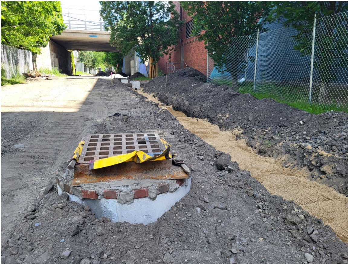
Catch basins have been raised up to correspond to the future elevation of the path
