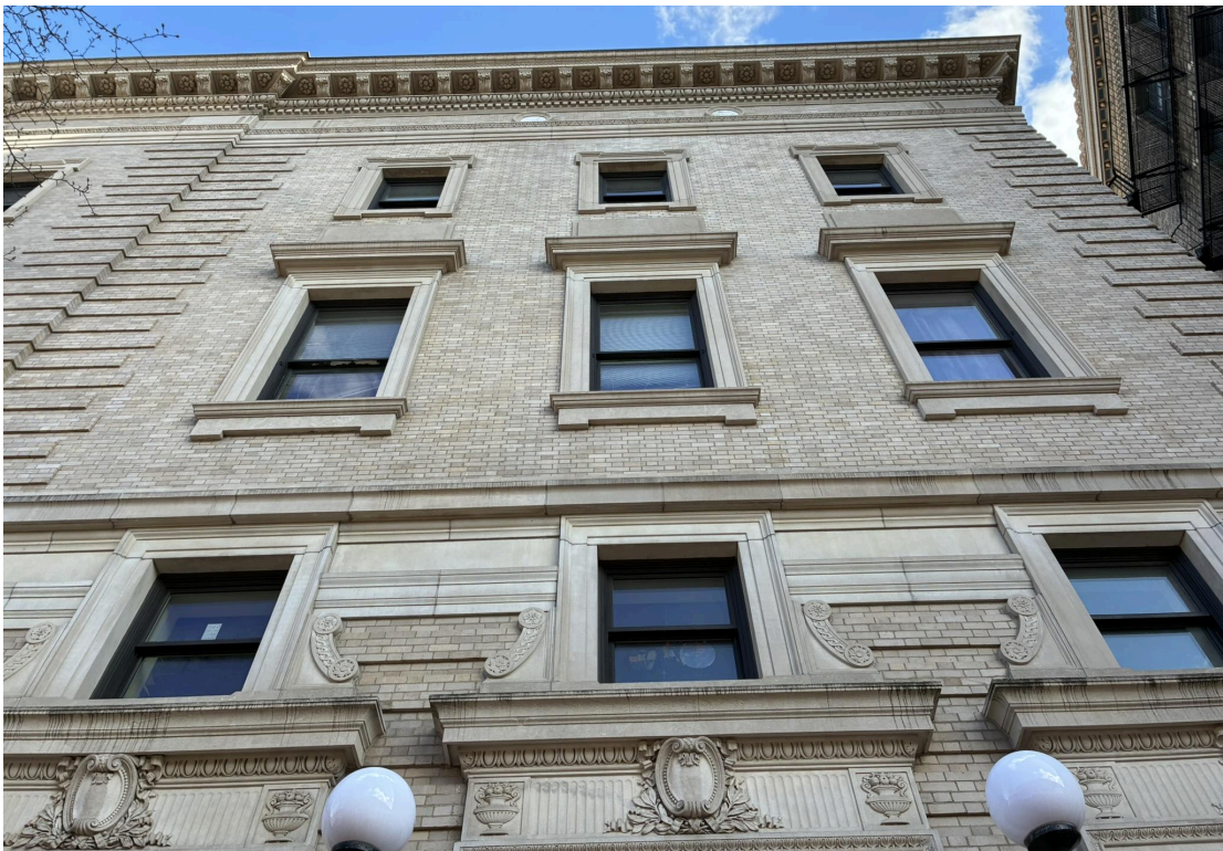
Figure 10. Detail of New England Conservatory facade on Huntington Avenue. March 2026 by Jennifer Gaugler.
