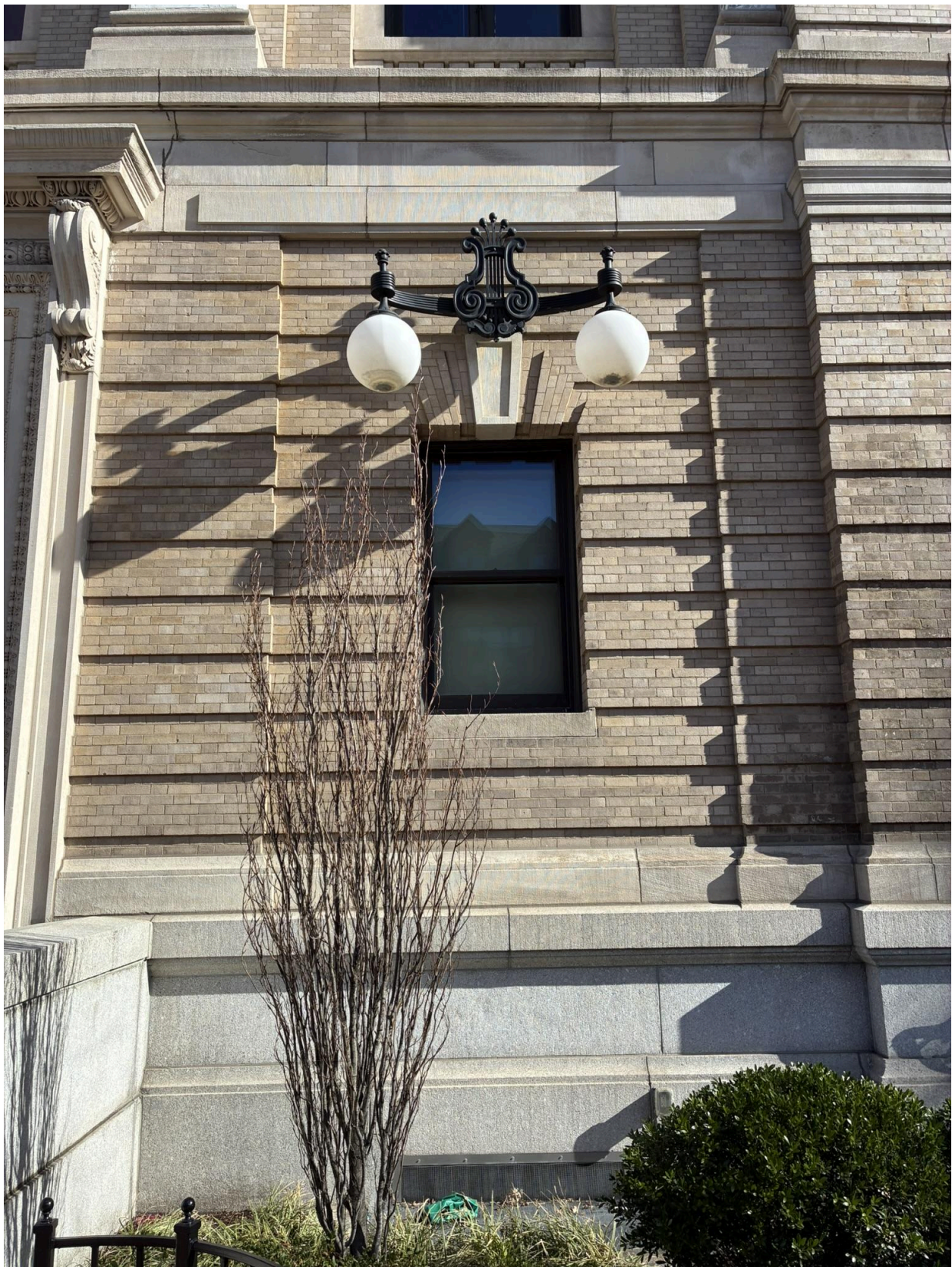
Figure 12. Detail of non-original light fixture adjacent to entrance on Huntington Avenue (compare to Figure 24 ). March 2026 by Jennifer Gaugler.
